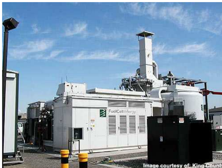
Figura 1.16 – Impianto da 1 MW a Renton, King County, Washington (FuelCell Energy).
