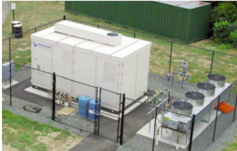
Figura 1.14 – Impianto da 200kW a South Widsor, Connecticut (UTC Power).
