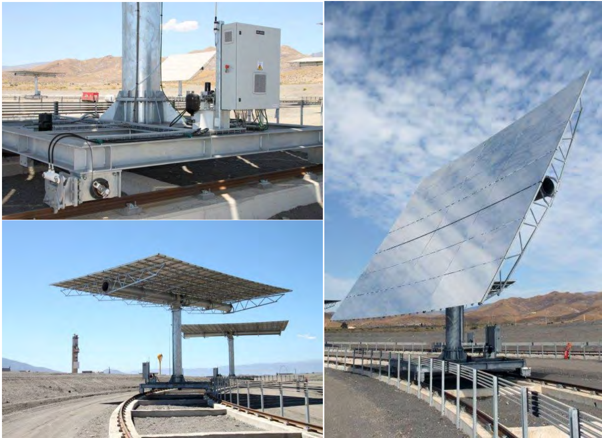
Figure 4-4: heliomobile details at CTAER. Up left, mobile platform and wi-fi control unit; down left rest position and rail; right, heliomobile under testing, fed by the power string.
