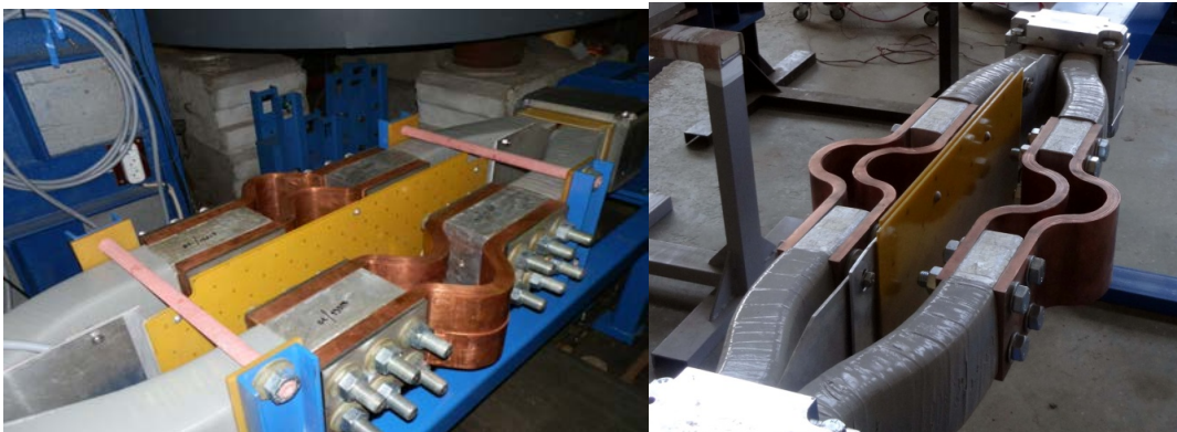
Figure 3.19: PF Busbar and CC Busbar thermal expansion compensator [8]
