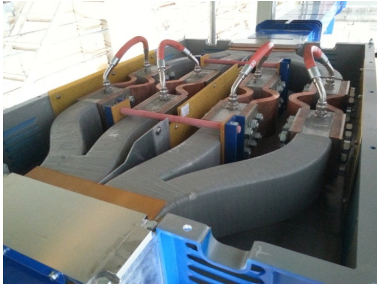
Figure 3.20: TF Busbar thermal expansion compensator and water cooling connections between the Busbars [8]
