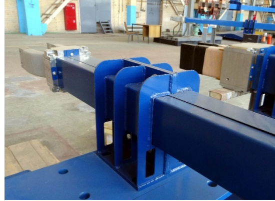
Figure 3.18: Supports of the CC Busbar [8]
