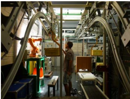
(a) The power & free conveyor.
