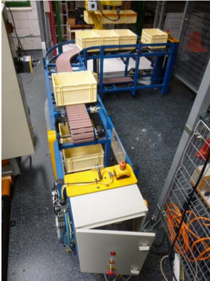
(a) View to the power & free conveyor.
