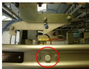
Figure 2.6: An inductive sensor of the power & free conveyor.
