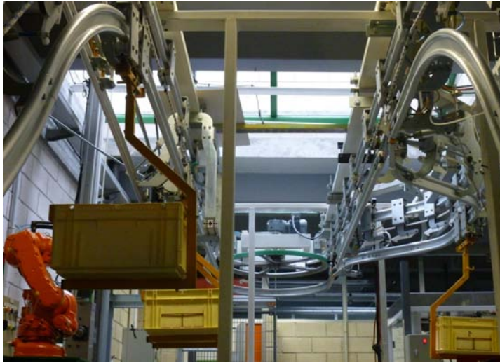
Figure 3.1: Higher floor (with a path deviation) in the area of power & free conveyor.
