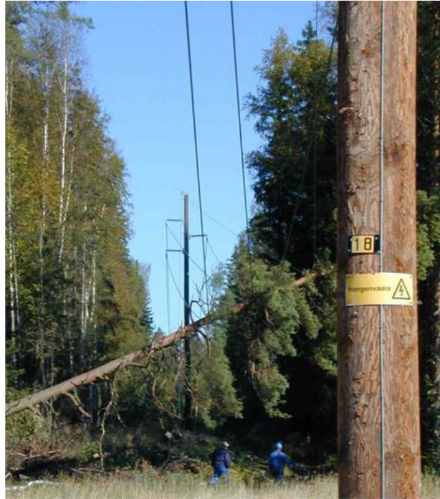
Figure 2.1 A tree fallen on a covered conductor line.
