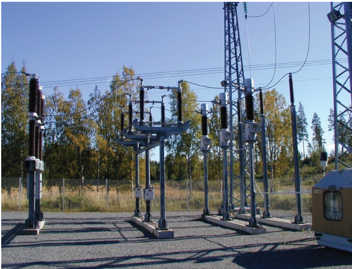
Figure 4.11 Switches, disconnector, earthing disconnector, PD sensors and support insulators located in Noormarkku 110/20 kV substation.
