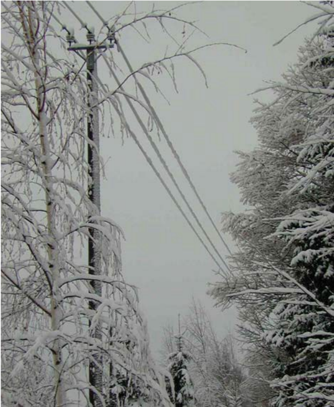
Figure 1.2 Covered conductor line under freezing condition.
