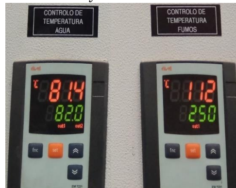
Figure 5.5.2 – Biomass boiler's temperature sensors
