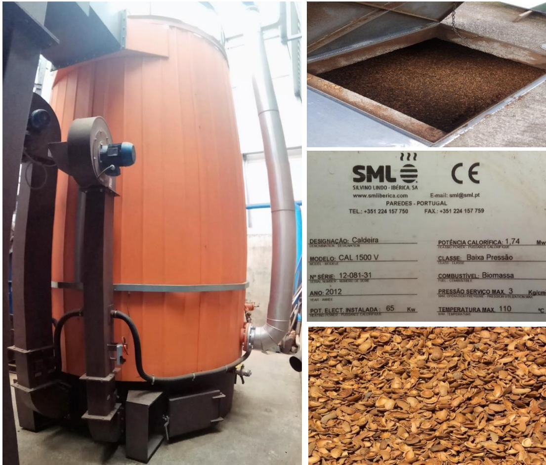
Figure 5.5.1 – Biomass, Biomass boiler's specifics, amonds and olive waste, biomass boiler
