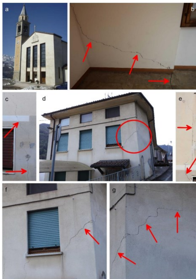
Figure 37: Pictures of Rovegliana Church (a) and one of the most damaged buildings in Cappellazzi district (c–g). In (b), a large crack in the portico of the church is shown [6]
