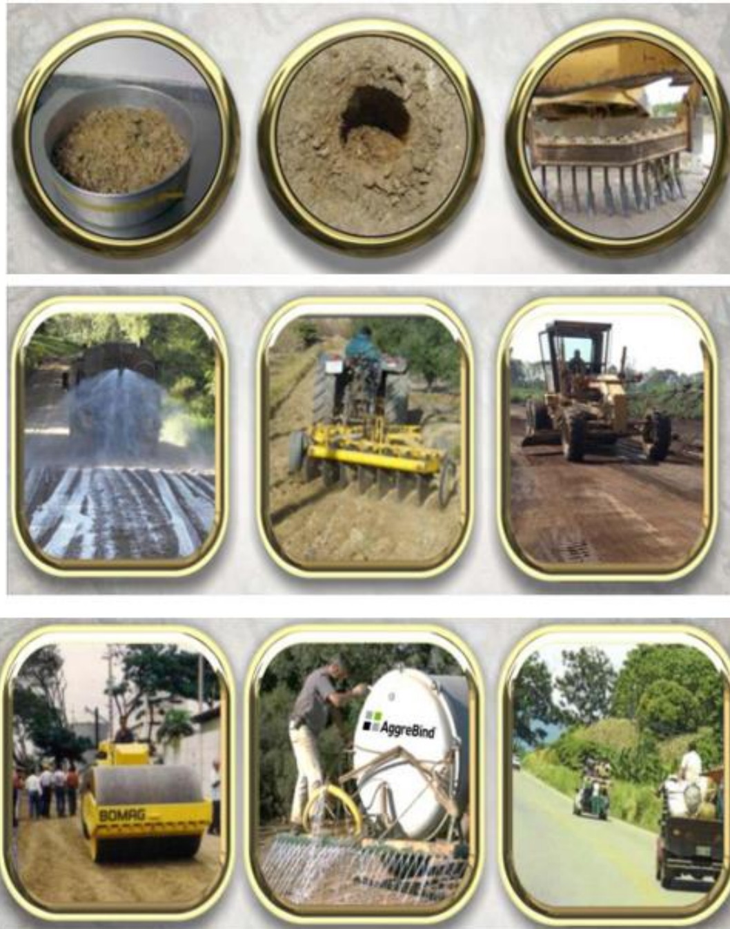
Figure 2. 4. In-situ stabilization process of rural tracks using the AggreBind product, ( www.aggrebind.com. , visited on 28/02/2021)
