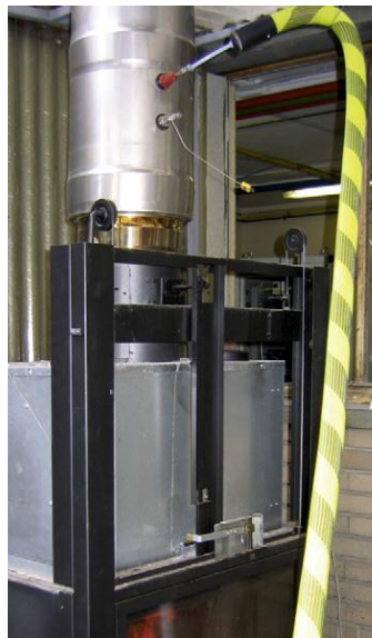
Fig. 1.2: Monitoring system of the temperature and the exhaust gases composition at the stove chimney (Bensaid, 2012)
