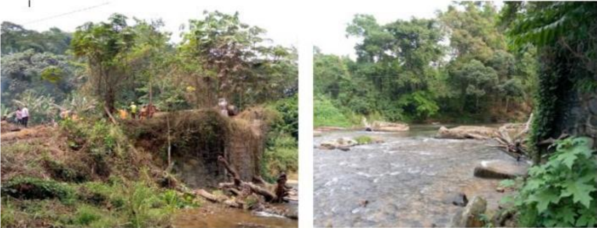
Figure 3.2. State of the two abutments of the old bridge
