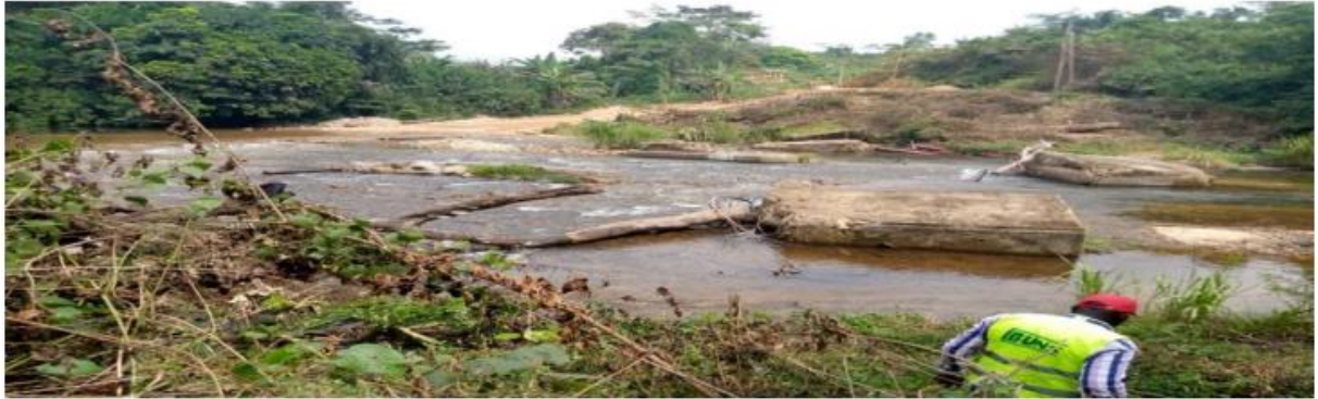
Figure 3.3. Debris of the previously collapsed bridge on the Mahe river
