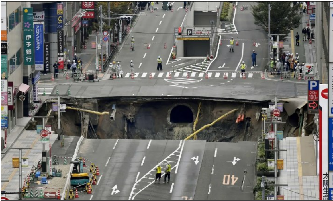
Figure 2.20 Sinkhole occurred in Fukuoka, Japan. Source: (Japan: Repaired Fukuoka Sinkhole Sinks Again - BBC News)
