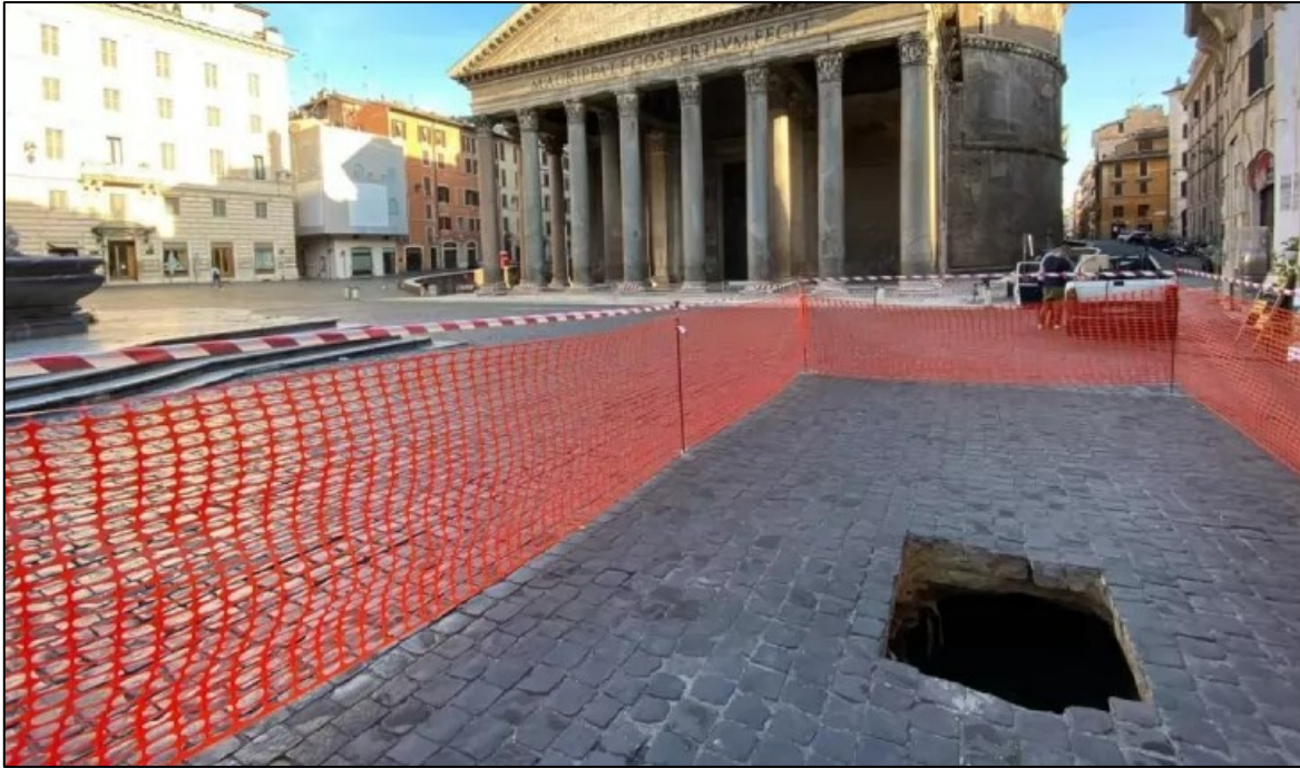
Figure 2.21 Sinkhole appeared in front of the Pantheon, Rome. Source: (Rome: Sinkhole Opens up in Front of Pantheon - Wanted in Rome)
