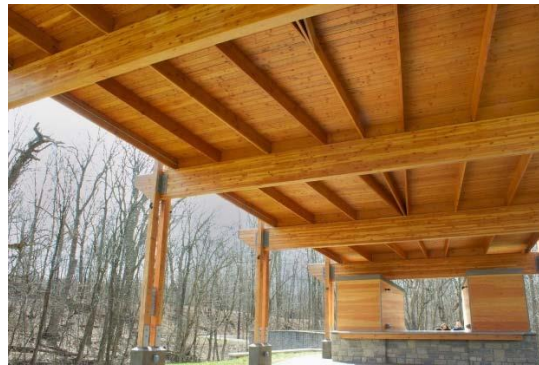
Figure1.13. Timber slab construction ( http://www.architectmagazine.com/techology/somtests a mass timber composite system for high rise construction and explores a steel option, 2012)
