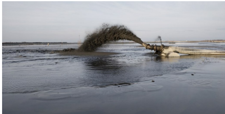
Figure 2.10. Disposal of dredged soil and water mixture at Le Sorelle-B site via pipeline and hydraulic pumping.
