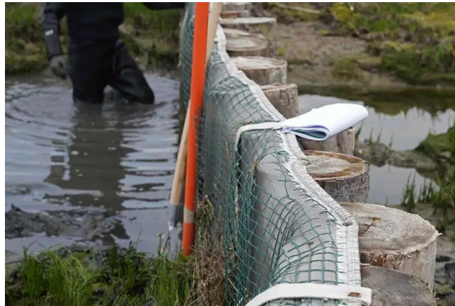
Figure 2.2. Wooden poles and geotextile sheets as containment structure for a salt marsh restoration project.
