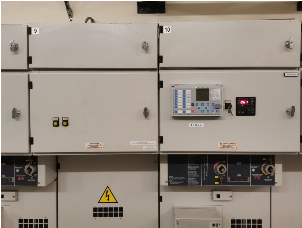
Fig.16 Photographic survey of generator protection
