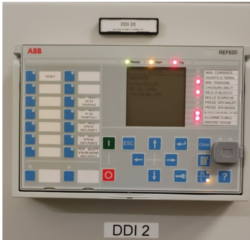
Fig.15 Photographic survey of interface protection relay
