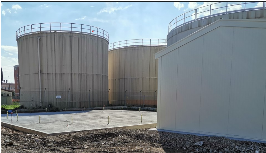
Fig.10 Photographic survey of two domestic water tanks (on the left and in the middle) and of chilled water tank (on the right).
