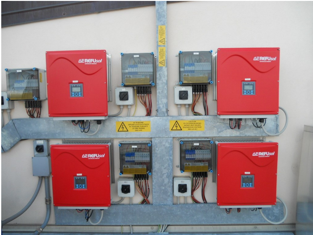
Fig.9 Photographic survey of PV inverters
