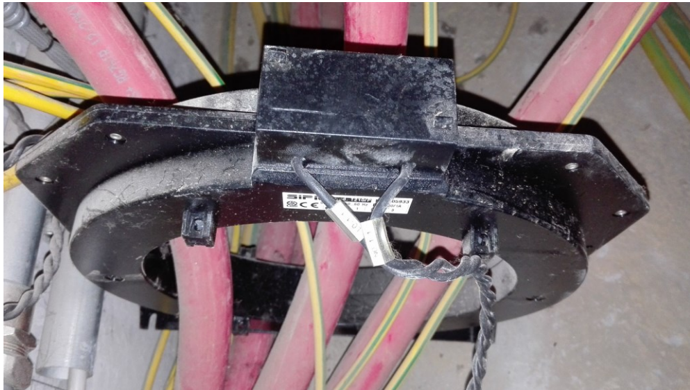
Fig.14 Homopolar transformer photographic survey
