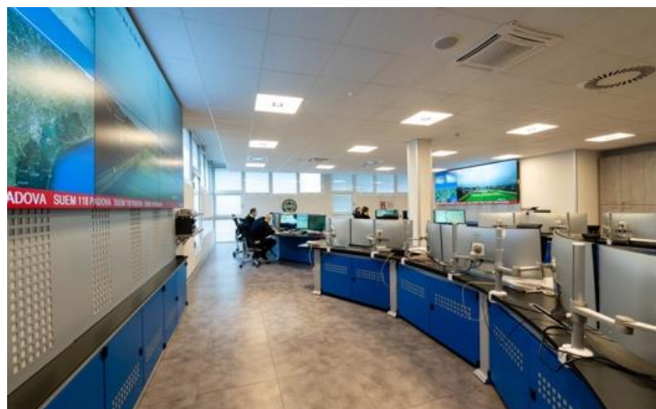
Figure 2: Padua EMS Dispatch Control Room
