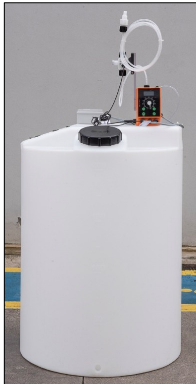
Fig. 4.51 Anti-scale product dosing pump with its relative tank
