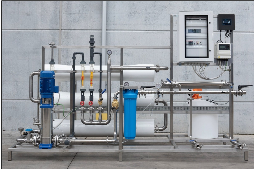
Fig. 4.52 Second reverse osmosis plant – forward view
