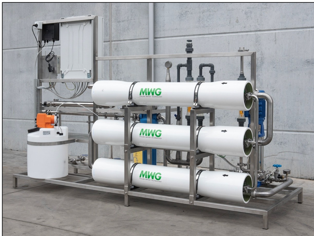
Fig. 4.53 Second reverse osmosis plant – backward view
