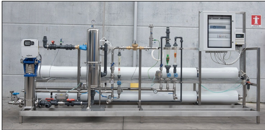
Fig. 4.33 First reverse osmosis plant – forward view
