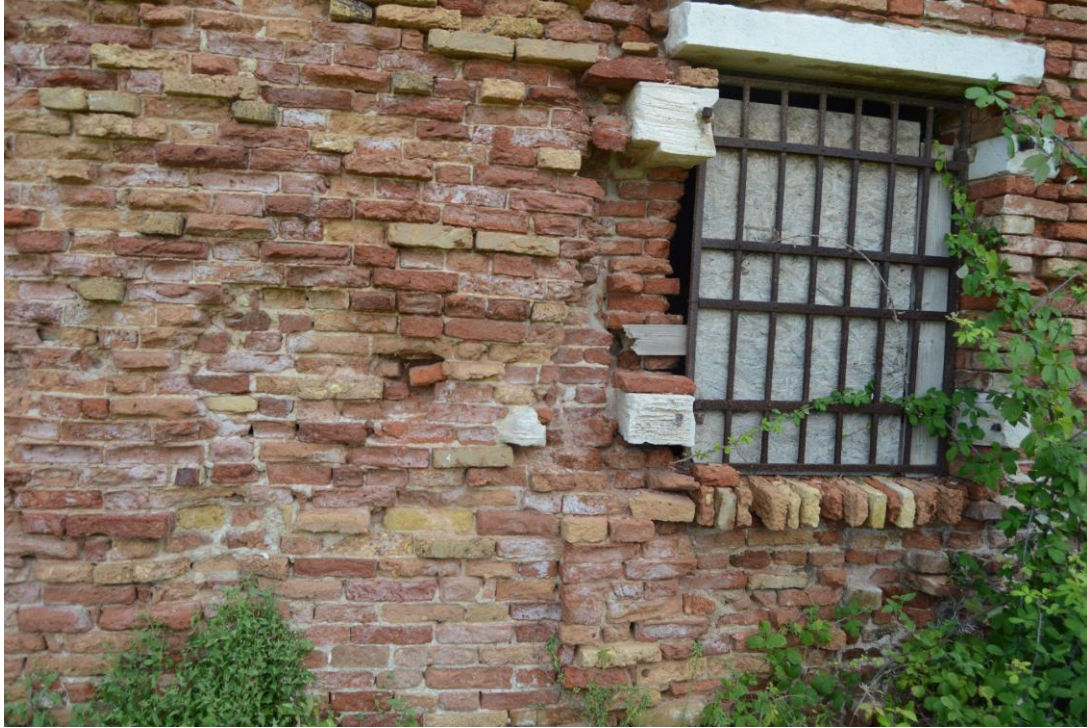
Figure 43. Chromatic alteration on the W façade of the Generalato.
