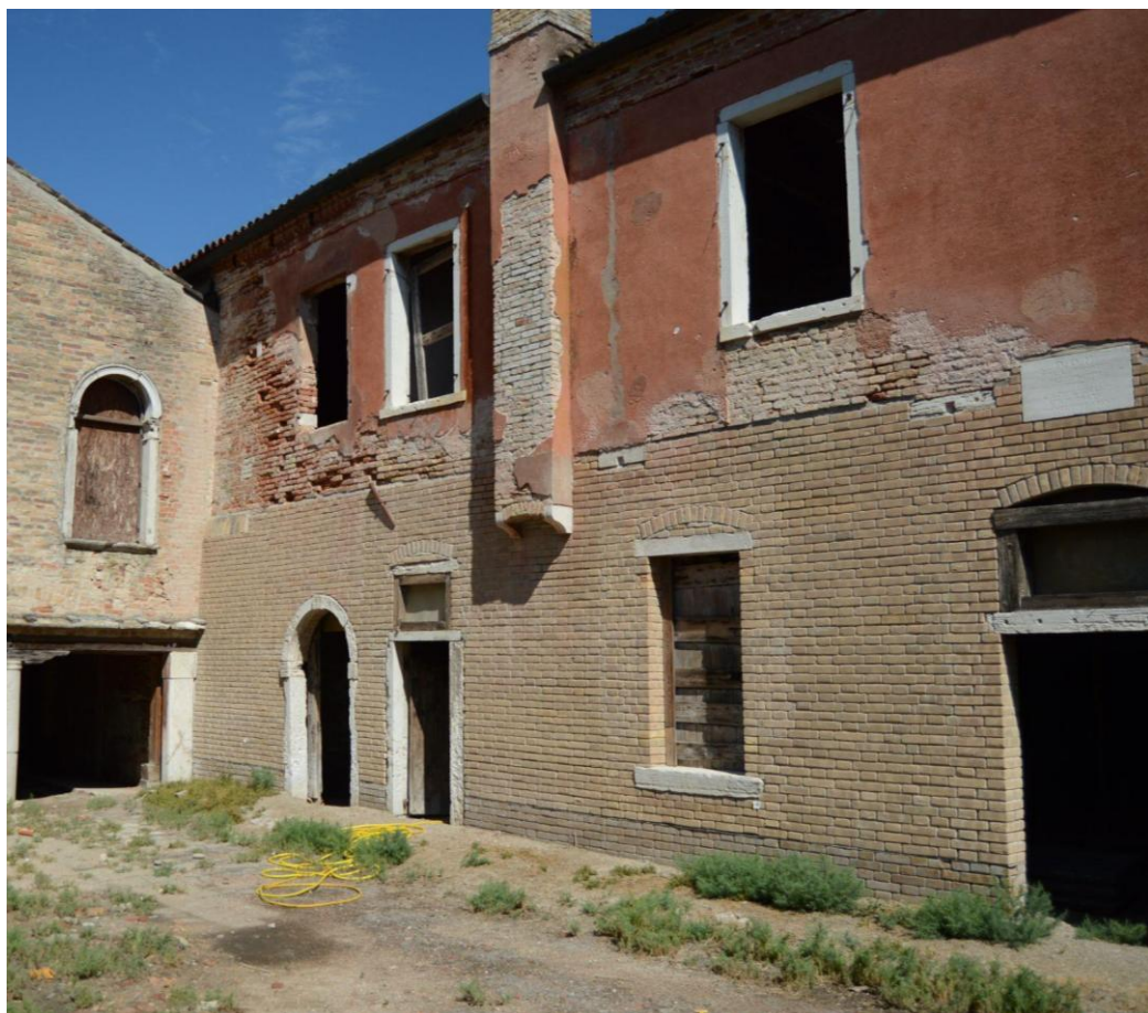
Figure 28. View of the southern façade of the Generalato, after the restoration of 1994.
