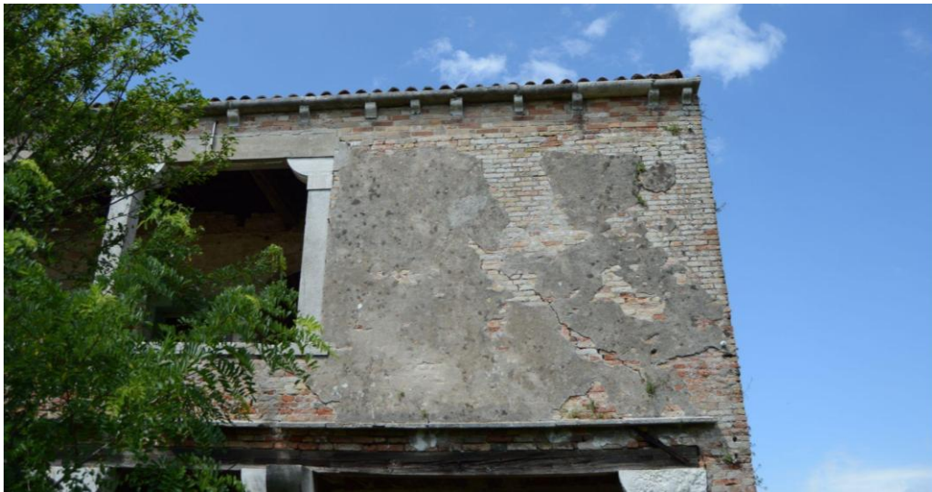
Figure 39. Plaster detachment on the E1 façade of the Generalato.
