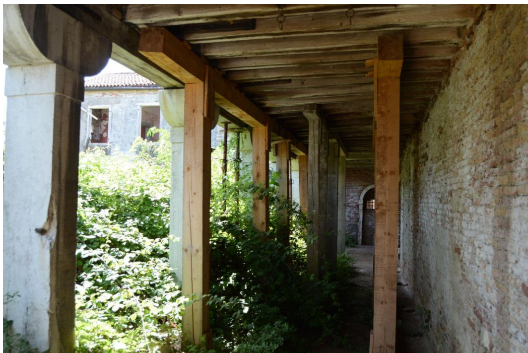
Figure 69. Shorings in the loggia of the Generalato.
