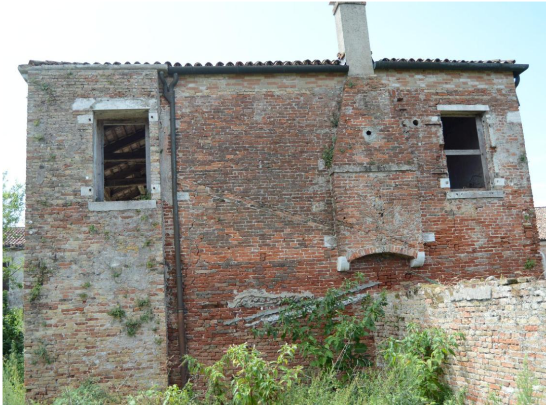
Figure 41. N1 façade of the Generalato, where a rusted downpipe is located.
