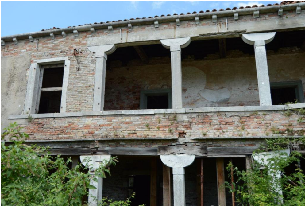
Figure 45. View of the E1 façade of the Generalato, displaying wooden beams in an advanced state of decay.
