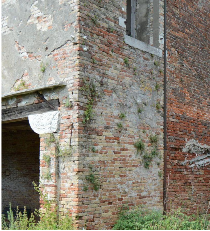
Figure 40. Biological colonisation on the E1 and N1 façades of the Generalato.
