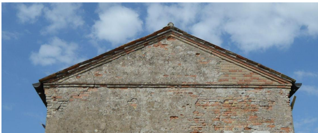
Figure 46. View of the E2 façade of the Generalato, where cracks can be noticed.
