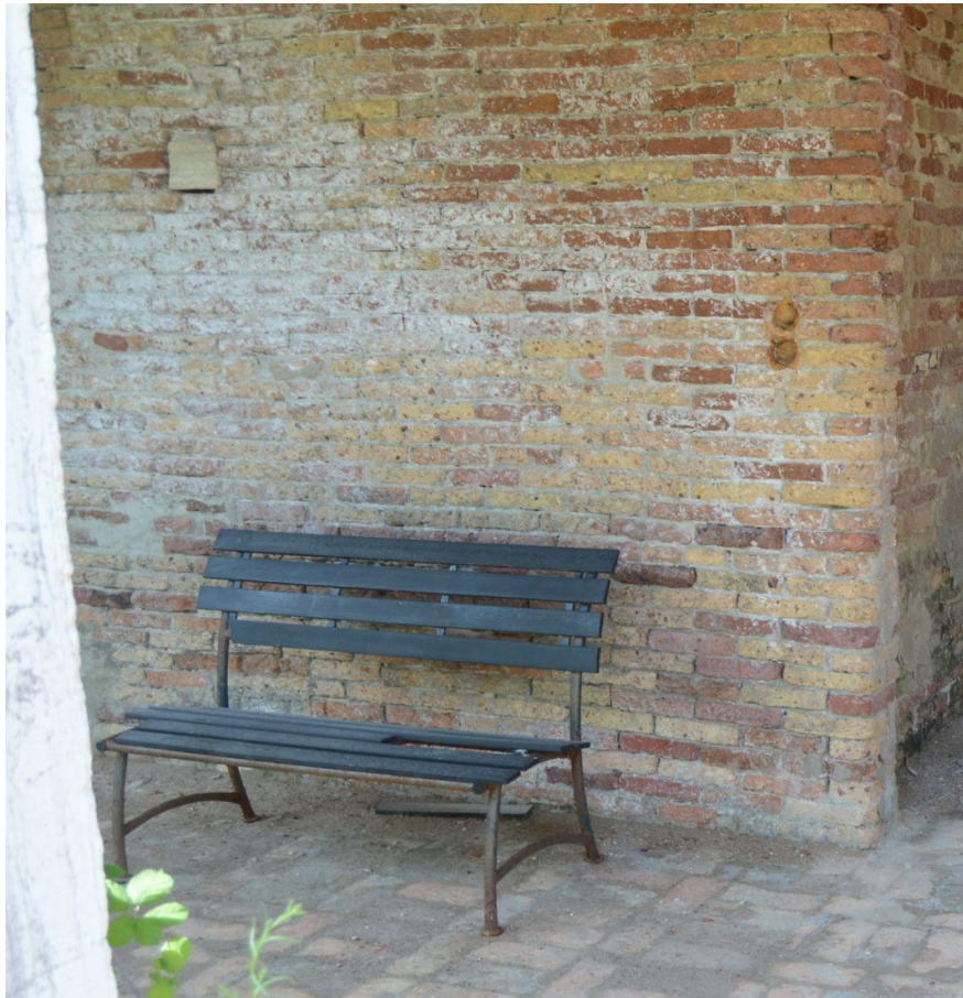
Figure 42. Efflorescence in an internal wall of the Generalato.
