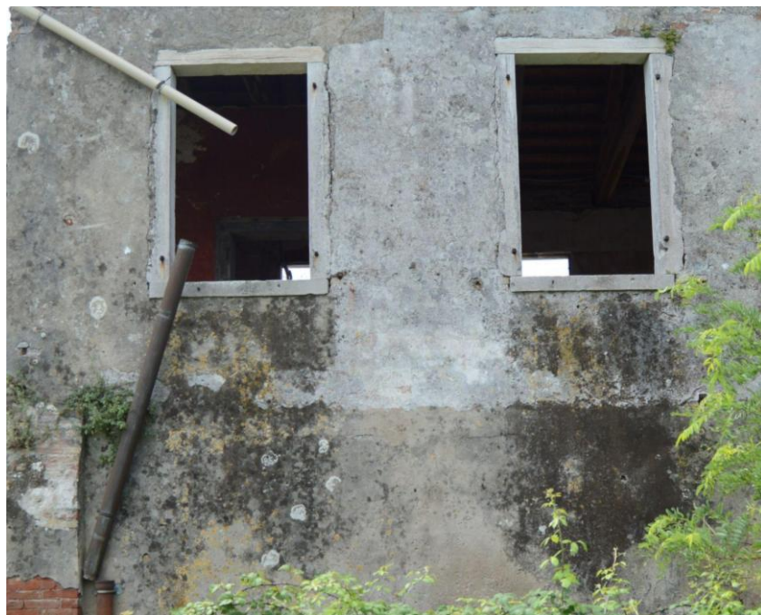
Figure 38. Mold growth caused by water infiltration on the N2 façade of the Generalato.
