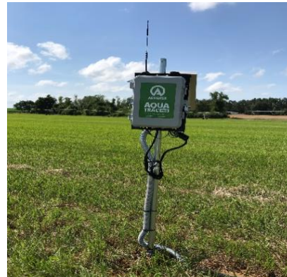
Figure 2-3. AgSense data logger mounted on 5 cm pipe approximately 3 m away from the probe.
