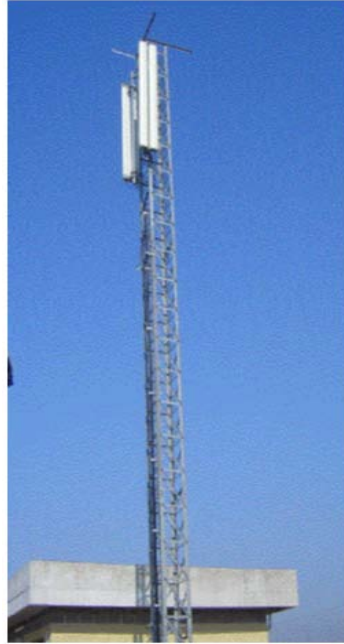
Figura 75 - Antenne BTS (Base Transceiver Station)
