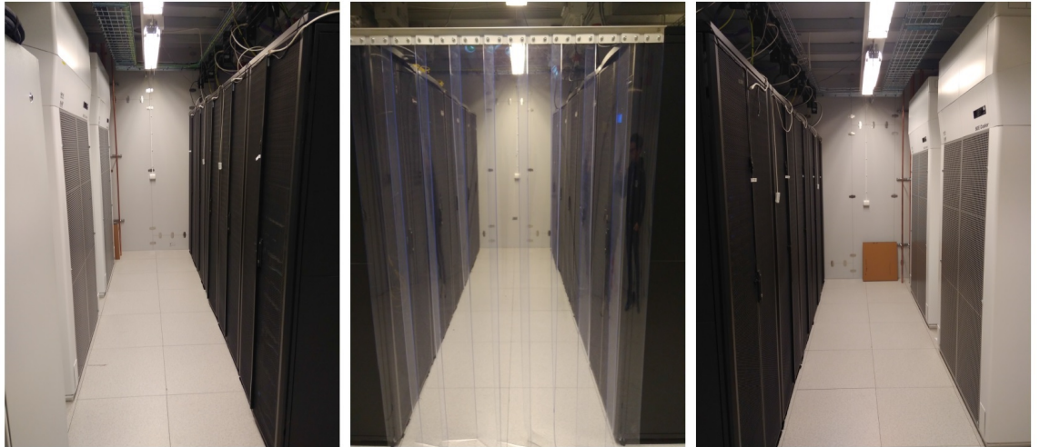
Figure 2.2: Example of a data center with hot aisle (central panel) and cold aisles (right and left panels) configuration.
