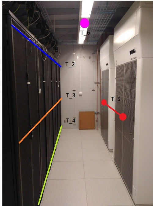
Figure 3.2: Clustered sensors within cold aisle. The image refers to the right side, but nothing change with the left side used.
