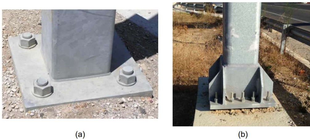
Figure 1.5. Conventional exposed tube column bases; (a) unstiffened tube base; (b) stiffened tube base (Kamperidis, 2016)
