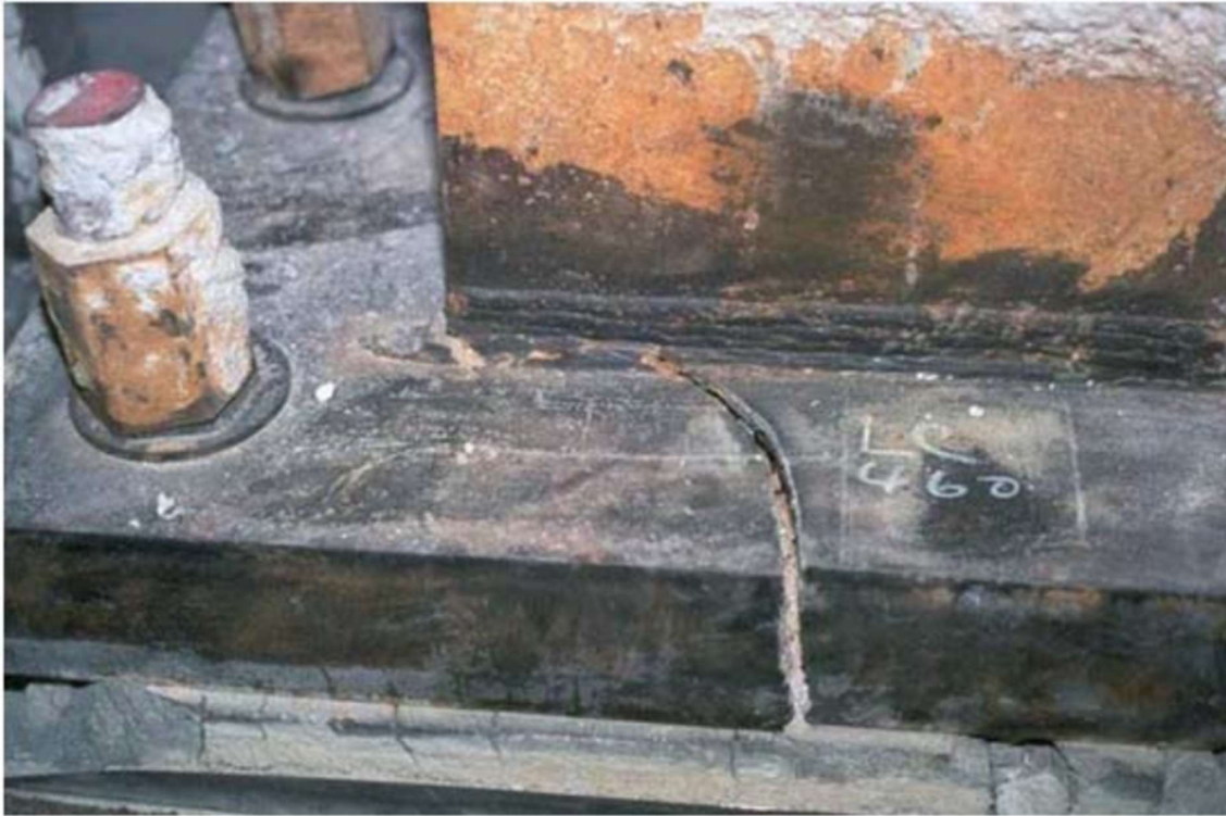
Figure 1.15. Close-up view of crack in a thick base plate (Lai et al., 2015)
