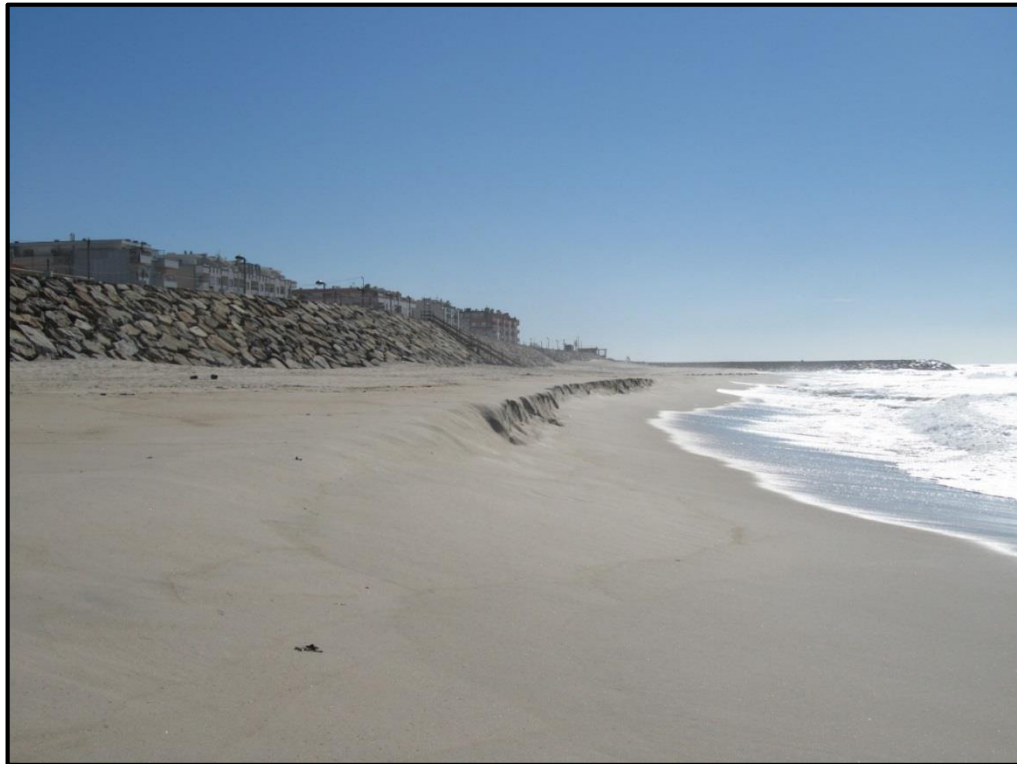
Figure 5.4. Vagueira seawall and Vagueira groin (North view). Site visit on October 2012.
