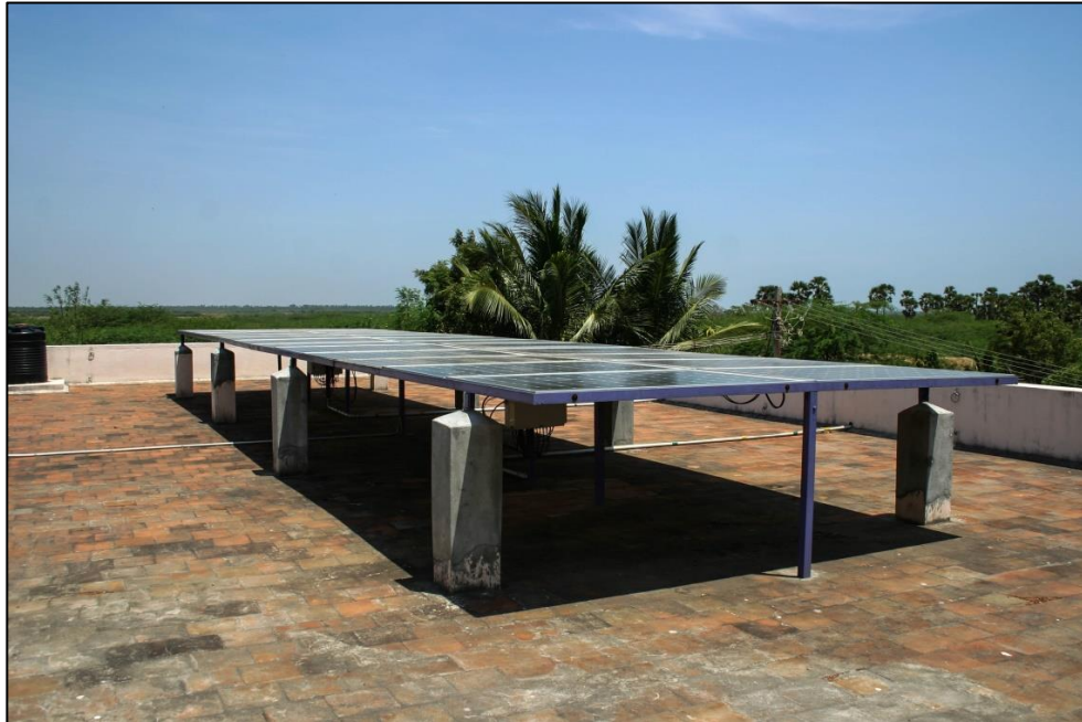
Figure 2.17: Photovoltaic panels on the roof of the storage
