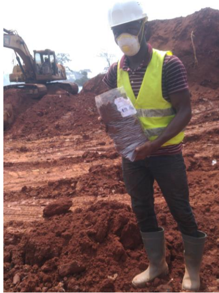
Figure 3. 10. Preparation of attacked soil by leachate.
