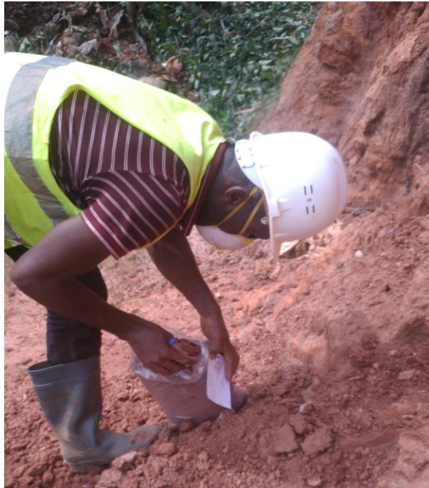
Figure 3. 9. Preparation of natural soil used for separation layer of wastes in a landfill.
