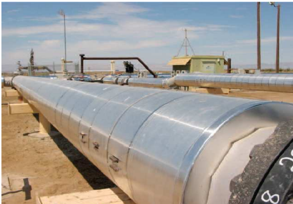
Figure 3 Super duplex 2507 turbine feed pipeline. [35]
