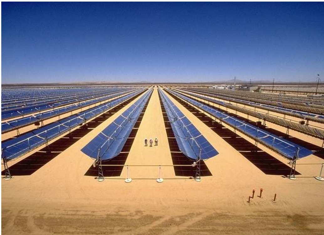
Figure 2: The Revolutionary Mojave's Desert Power Plant built by Luz International.
