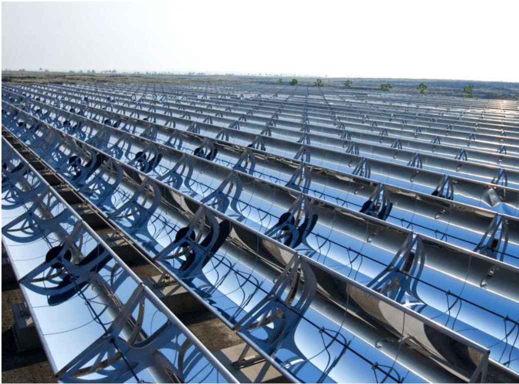
Figure 1.1: A parabolic trough collector system
