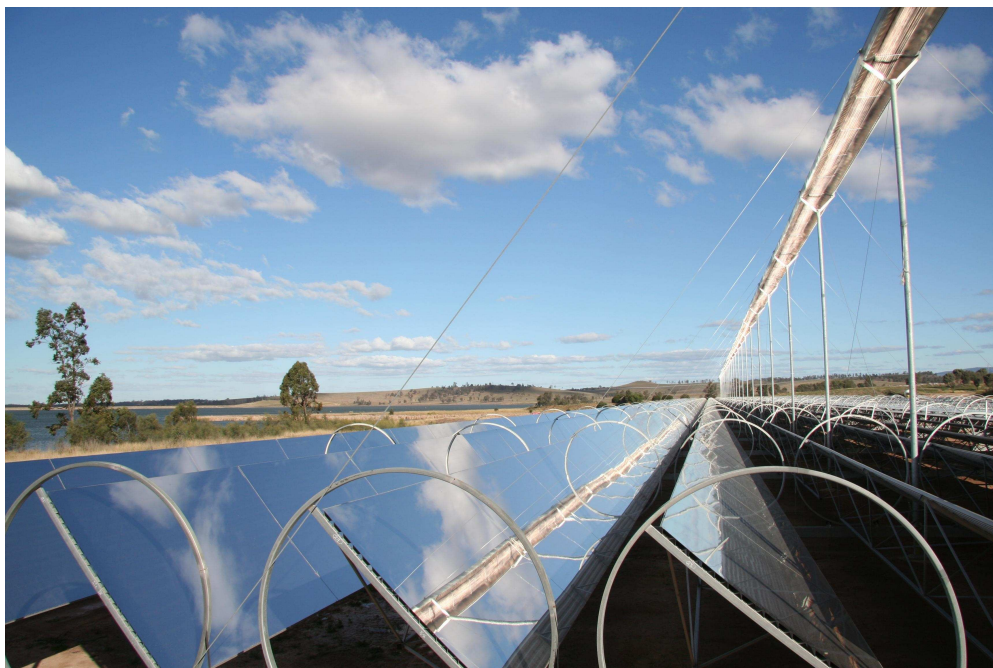
Figure 1.2: A Linear Fresnel collector system
