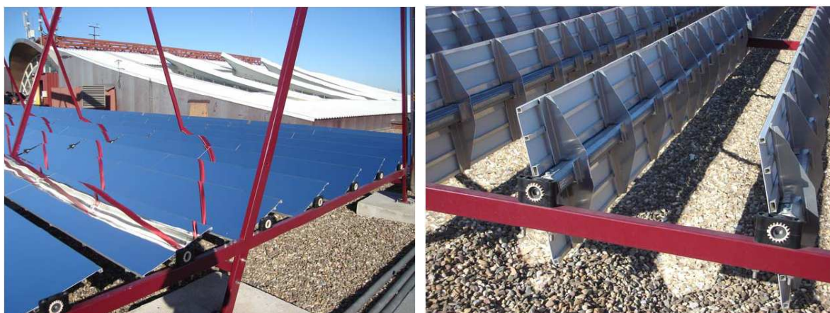
Figure 3.4: Reflective mirrors in operation (on the left) and in guard position (on the right).
