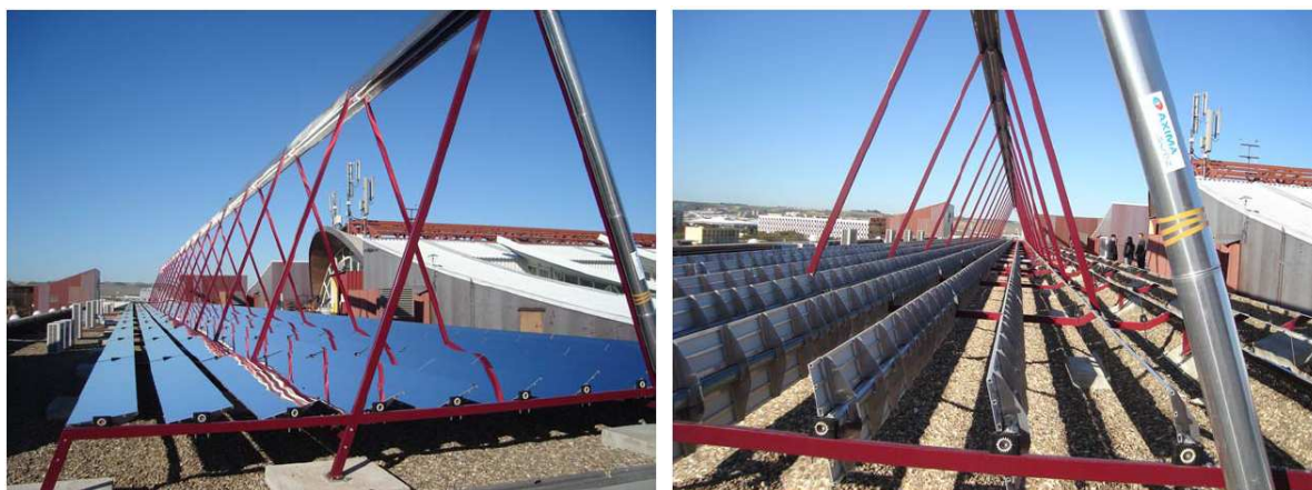
Figure 3.3: Global view of solar plant (on the left); a particular of steel structure (on the right).
