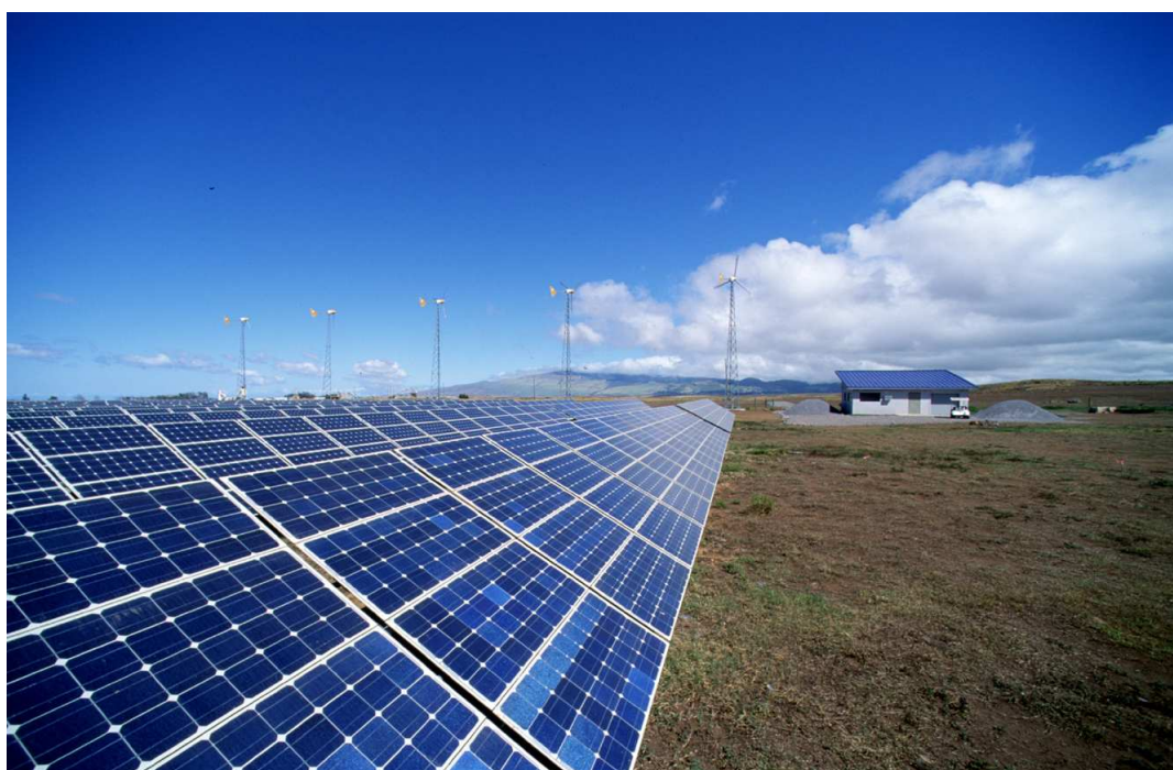
Figure 1.10: An example of Photovoltaic Arrays for energy production. The Europe biggest Photovoltaic Park is under construction in Italy, in the district of Rovigo, by the American SunEdison. The Park will have a surface of 850.000\text{ m}^2 (equal to 120 Football Fields) and a Power of 72 Megawatts.
