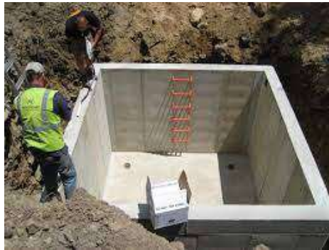
Figure 1. 7. Underground tank( www.indiamart.com )
