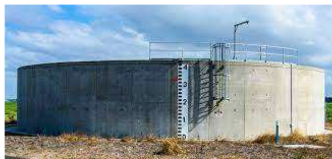
Figure 1. 5. Resting on ground tank( www.tuf-bar.com )
