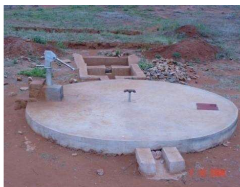
Figure 1. 13. Cylindrical cistern for surface rain water harvesting system (Alemu seifu,2011)
