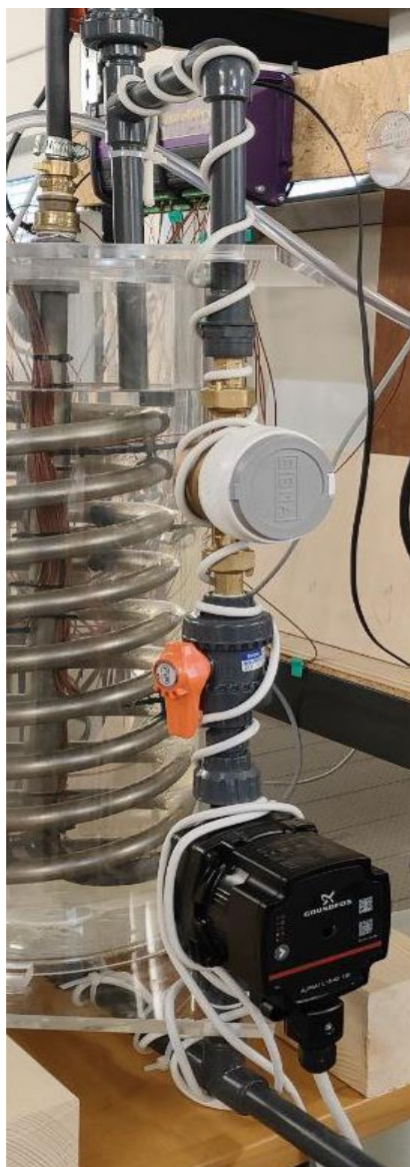
Fig. 2.4 - Heating cable wrapped around the external circuit
