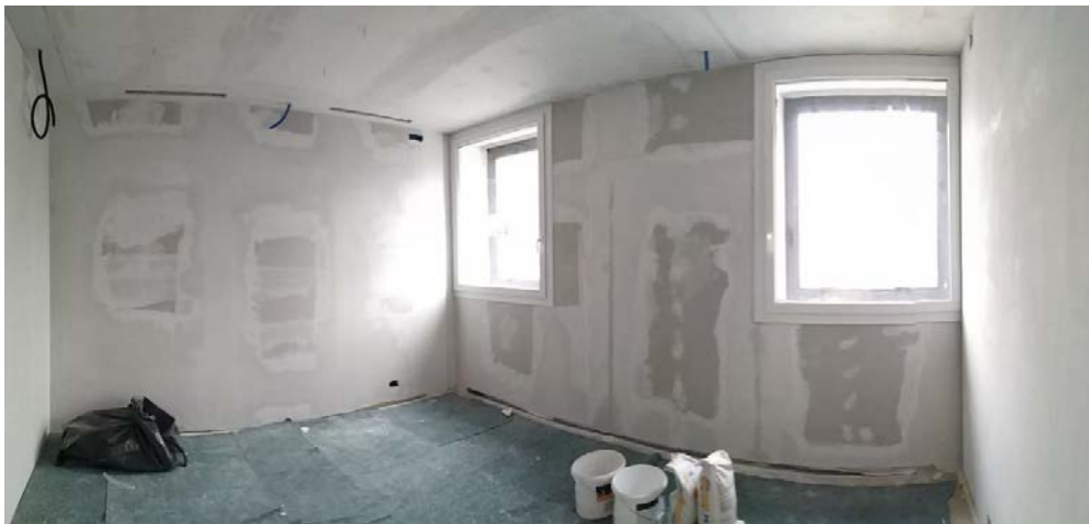
Fig. 55. North and east wall during the finishing of plasterboard and the painting of room
