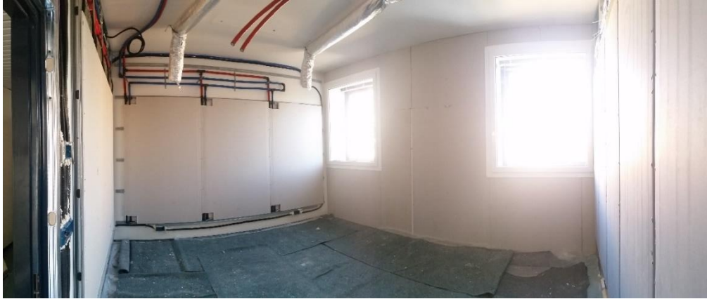
Fig. 53. North and east wall during the hydraulic and aeraulic connection and after the installation of windows and insulating material
