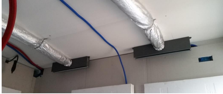
Fig. 43. Supply vents with plenums and ventilation ducts
