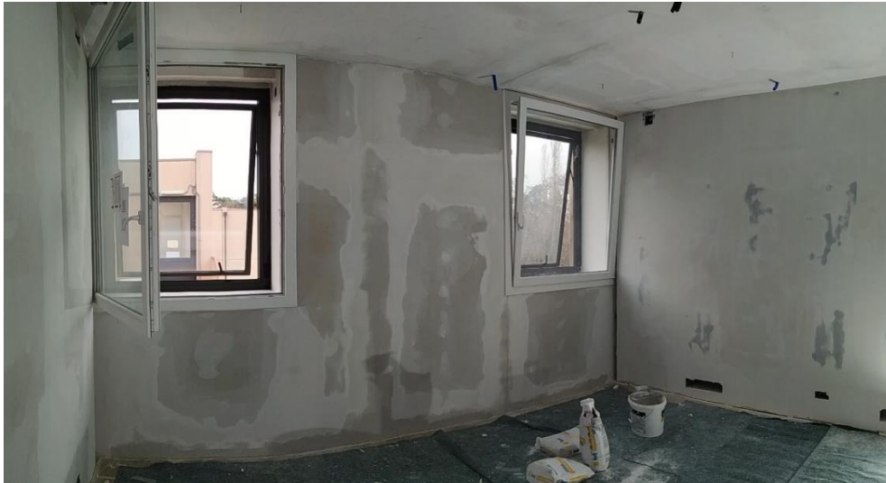
Fig. 56. East and south wall during the finishing of plasterboard and the painting of room
