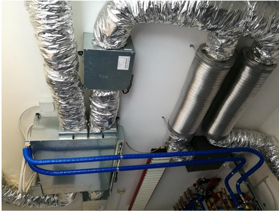
Fig. 48. Ventilation machine and aerulic ducts installed in the ceiling of the technical room
