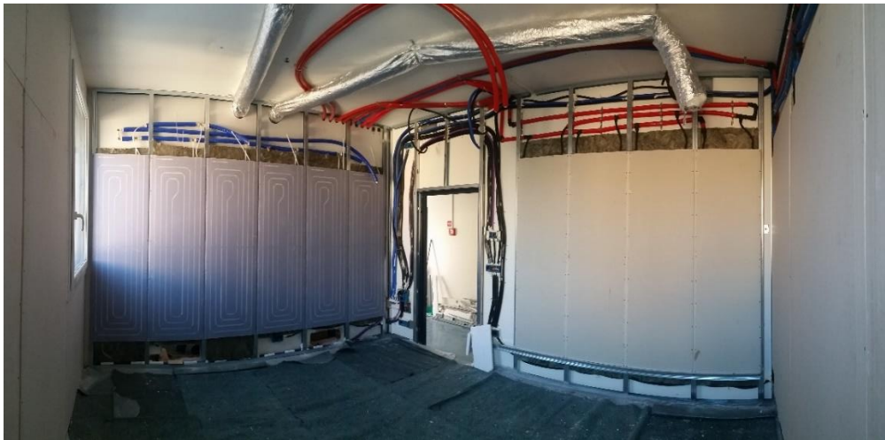
Fig. 54. South and west wall during the hydraulic and aeraulic connection and after the installation of windows and insulating material
