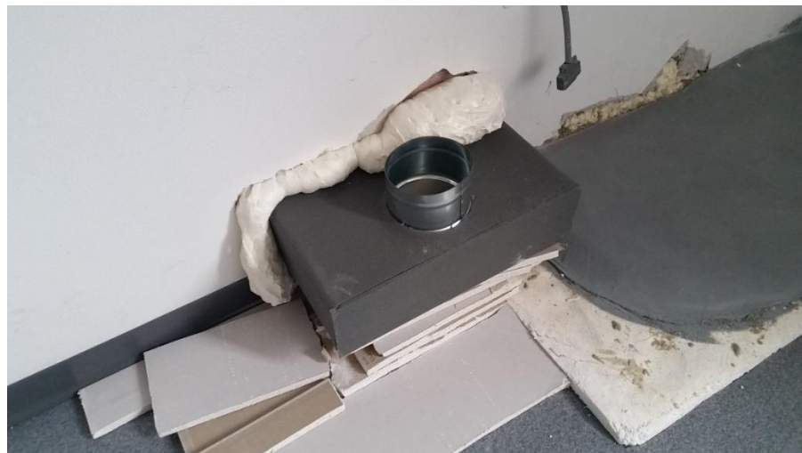
Fig. 45. Plenum of an extraction grid
