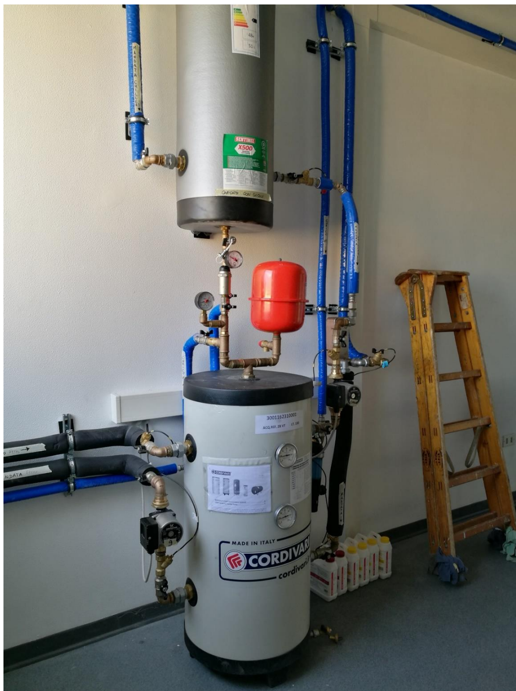
Fig. 64. Below: storage tank for chilled water. Above: chiller tank
