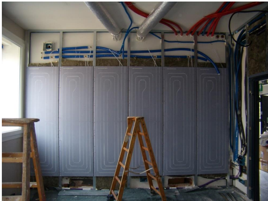
Fig. 38. South panels during the hydraulic connection and the insulation of hollow space
