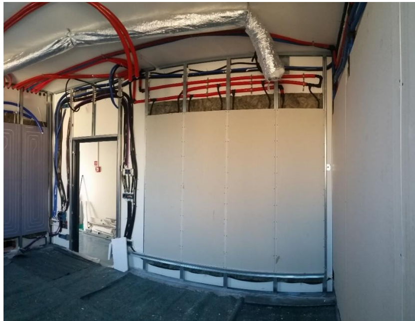
Fig. 42. West panels during the hydraulic connection and the insulation of hollow space
