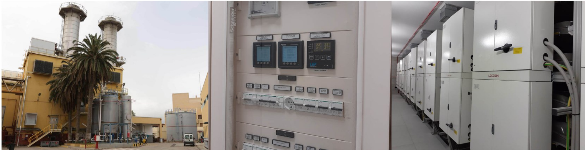
Melilla power plant and energy storage equipment
