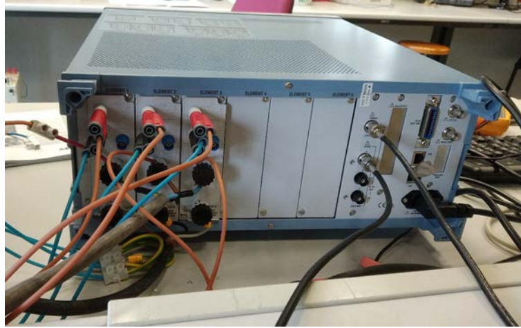
Figure 6.8: Power analyser wiring configuration (3P4W)
