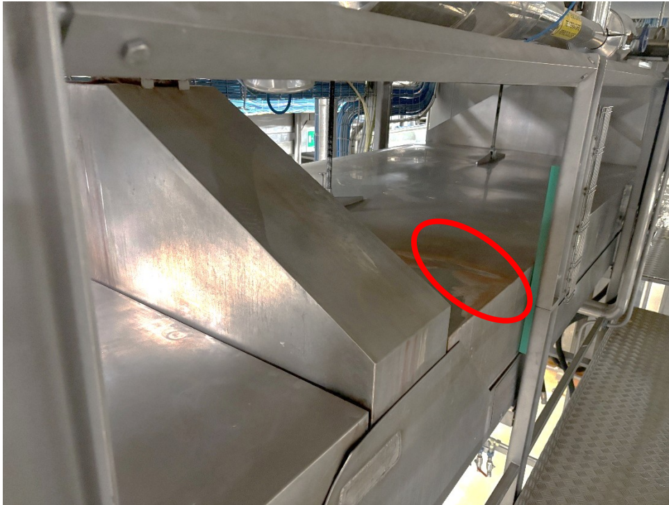
Figure 3.6: Corrosion on the upper surface of pasteurizer
