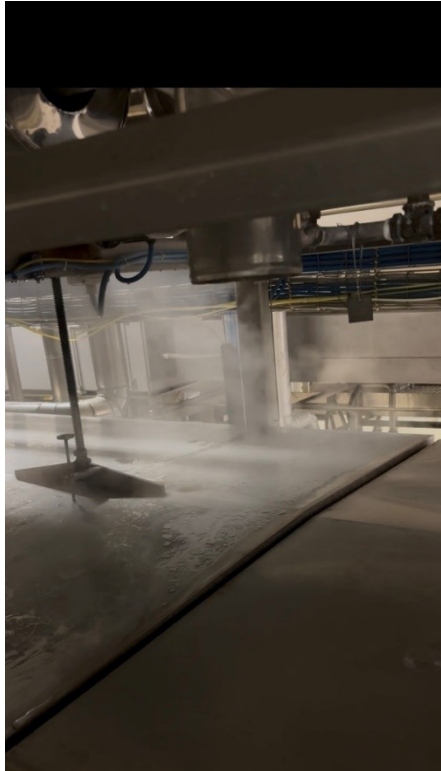
Figure 3.8: Direct steam leakage
