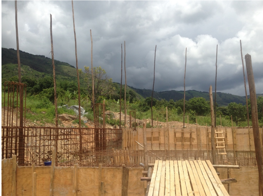
Figure 22 Powerhouse during the month of February
