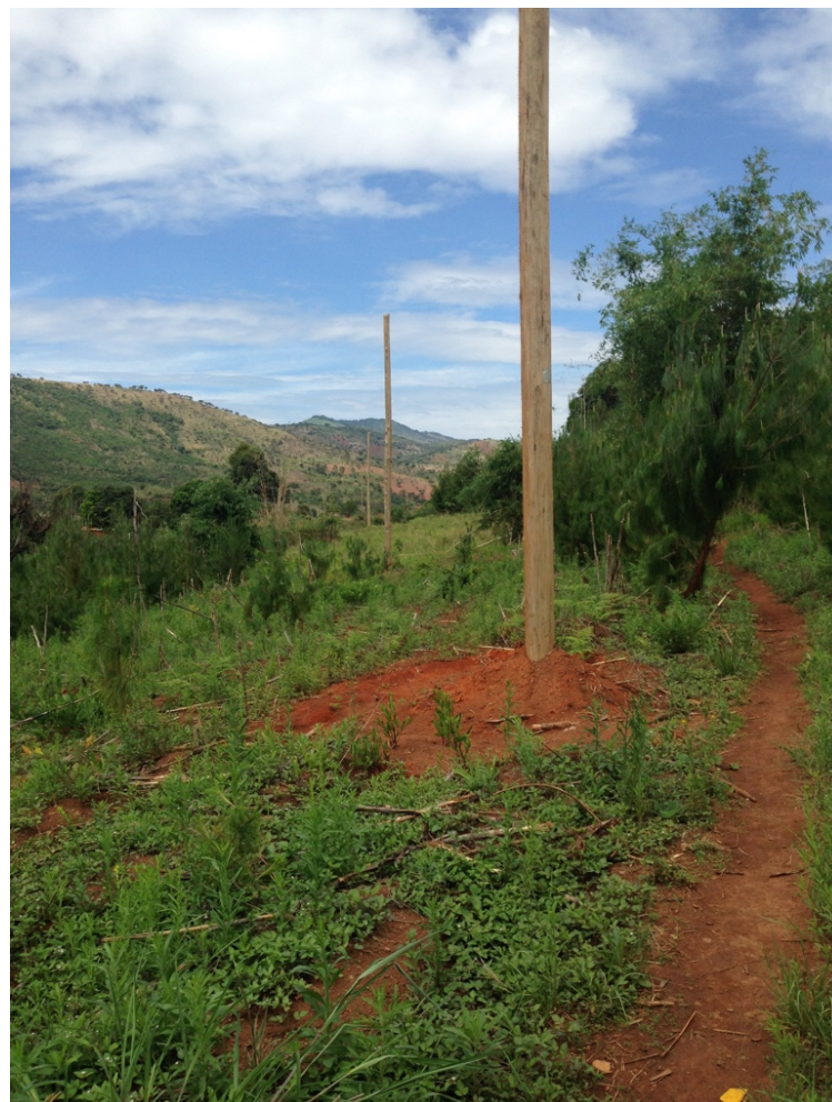
Figure 24 Power line during the month of December
