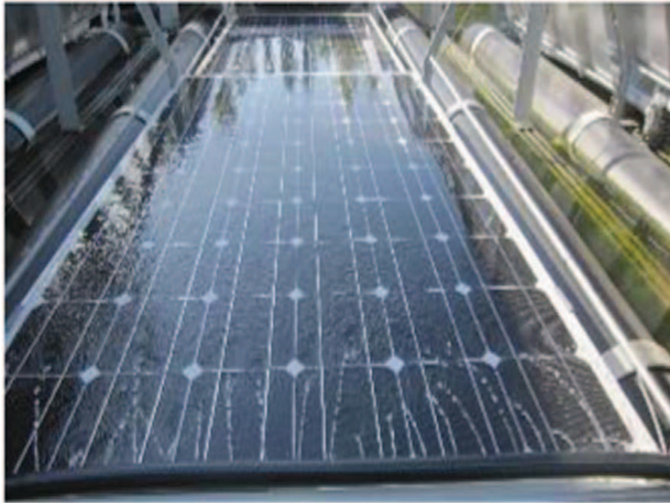
Figura 96 - Water Veil Cooling system
