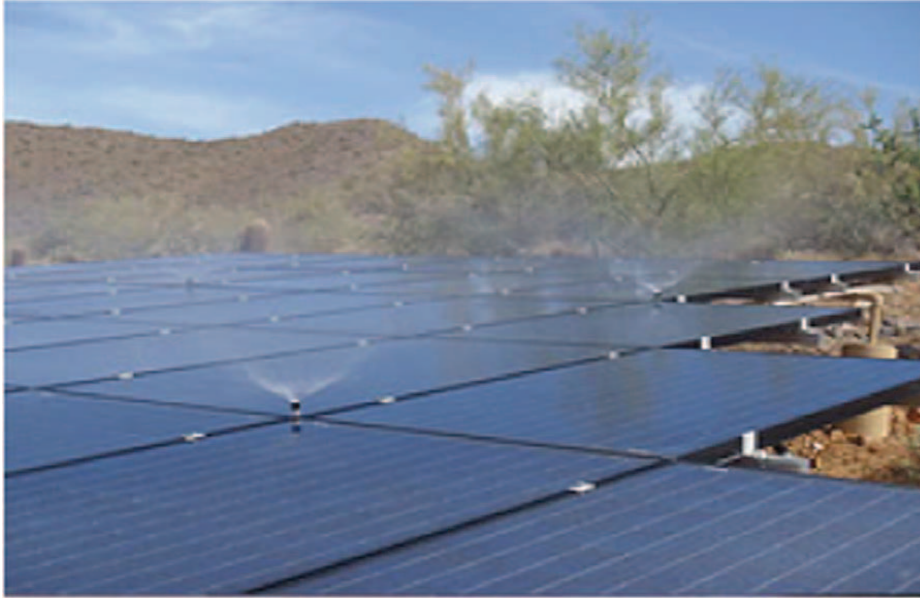
Figura 97 – Sprinkler Cooling System
