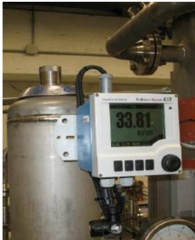
Figure III-15: Water conductivity sensor display.
