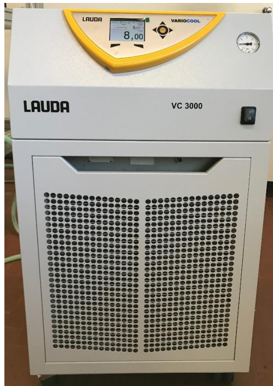
Figura 3-5 "chiller" LAUDA VC 3000.
