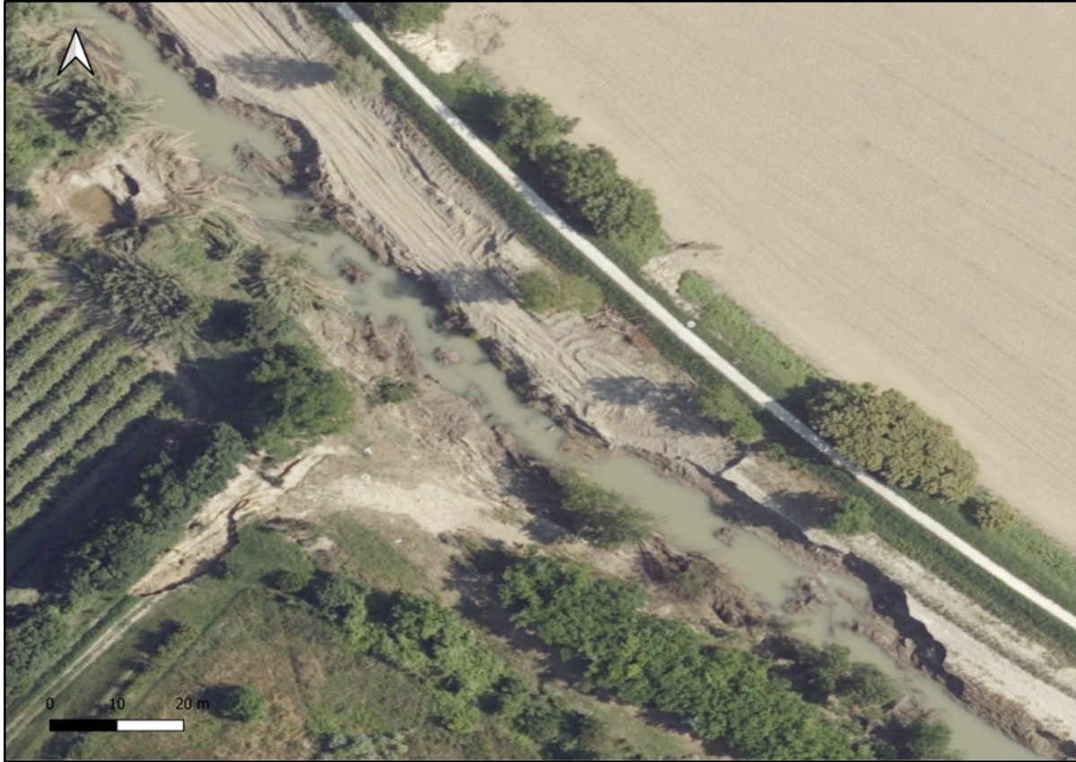
Figure 6.1: Observed bank erosion at meander section of Senio River
