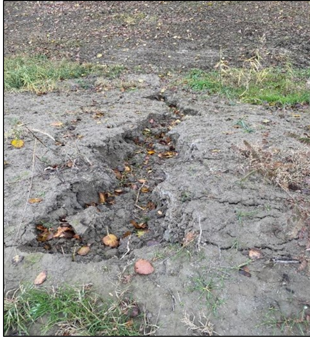
Figure 4.4 Erosion signs on levee body, Via del Tiglio site inspection
