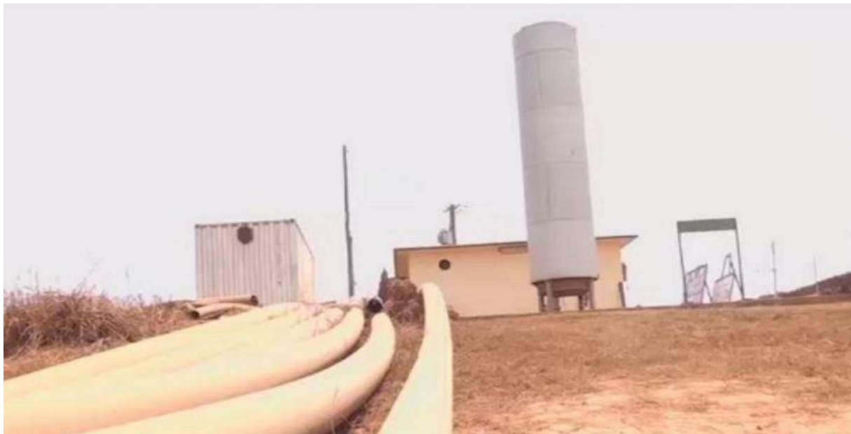
Figure 24: HYSACAM Biogas plant, Yaoundé.
