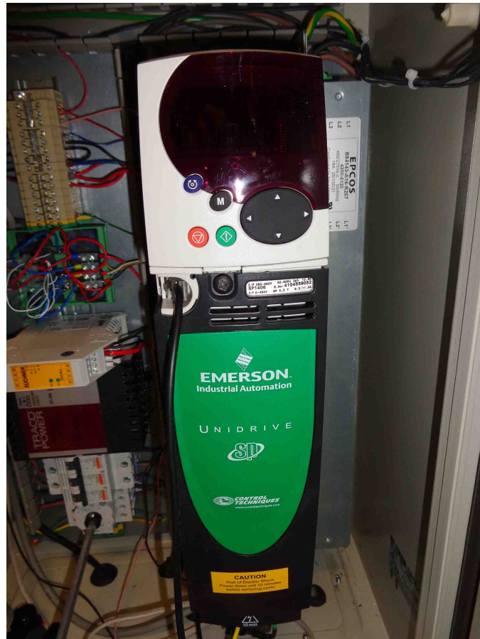
Figure 2.3: Emerson Control Techniques Unidrive SP1406
