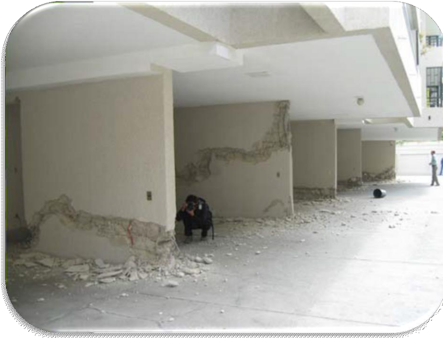
Figure 1.12. Failure of a Reinforced concrete shear wall due to slenderness (Carlos Videla, 2012)
