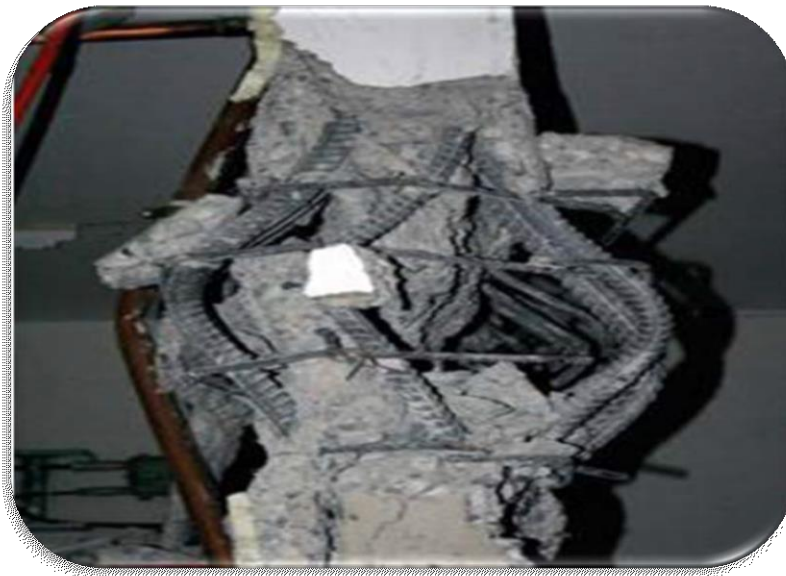
Figure 1.10. Failure of RC column due to poor detailing. (Carlos Videla, 2012)
