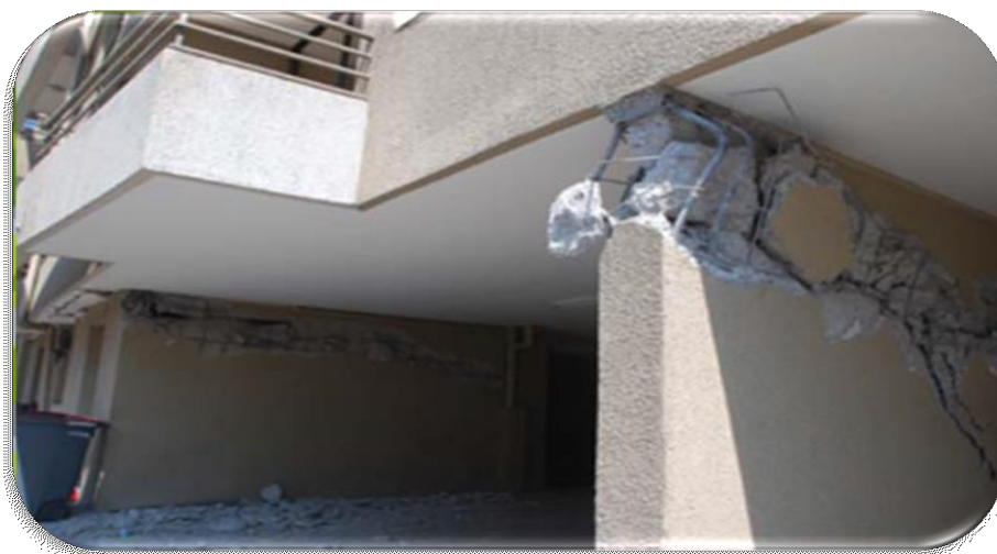
Figure 1.9. Failure of shear wall due to lack of confinement bars (Carlos Videla, 2012)
