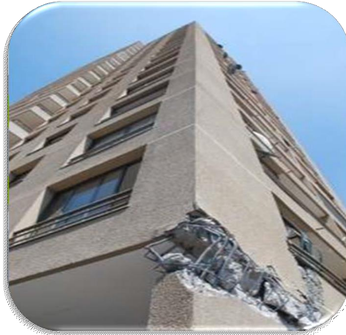
Figure 1.8. Soft floor failure on a reinforced concrete building. (Carlos Videla, 2012)
