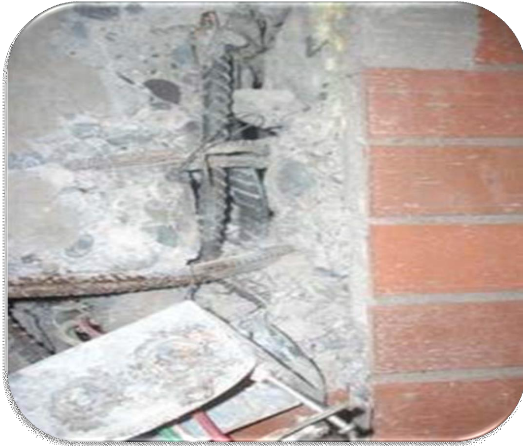
Figure 1.7. Splice failure on an RC building (Carlos Videla, 2012)
