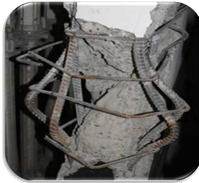
Figure 1.5. Concrete crushing and rebar buckling on a column element. (Carlos Videla, 2012)
