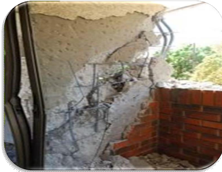
Figure 1.11. Shear failure of an RC wall (Carlos Videla, 2012)
