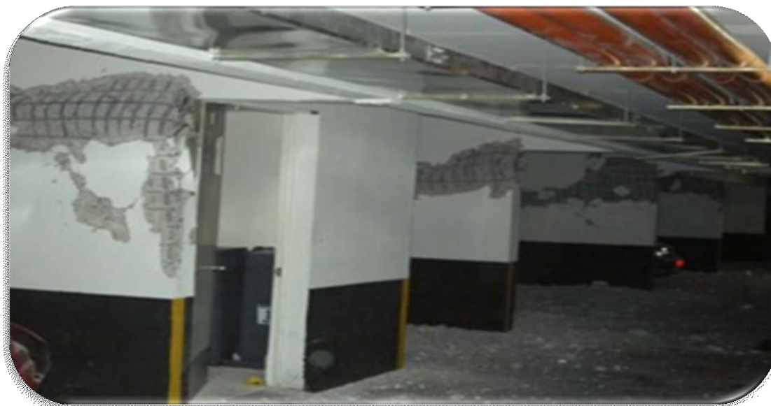
Figure 1.4. Flexural-compressional brittle failures on shear walls (Carlos Videla, 2012)
