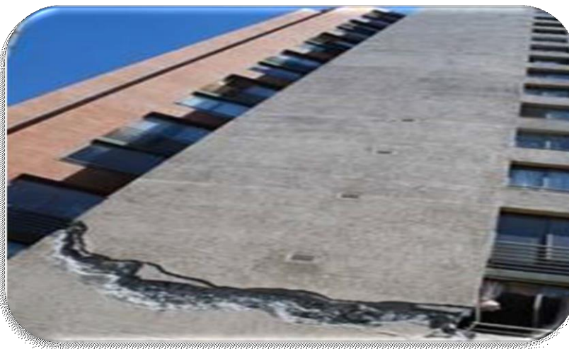
Figure 1.13. Indicate failure of a RC shear wall due to heavy loads (Carlos Videla, 2012)
