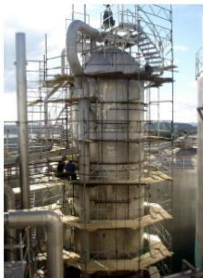
Fig. 7 Hydrogen peroxide reactor made in LDX 2101 (2006) [2]
