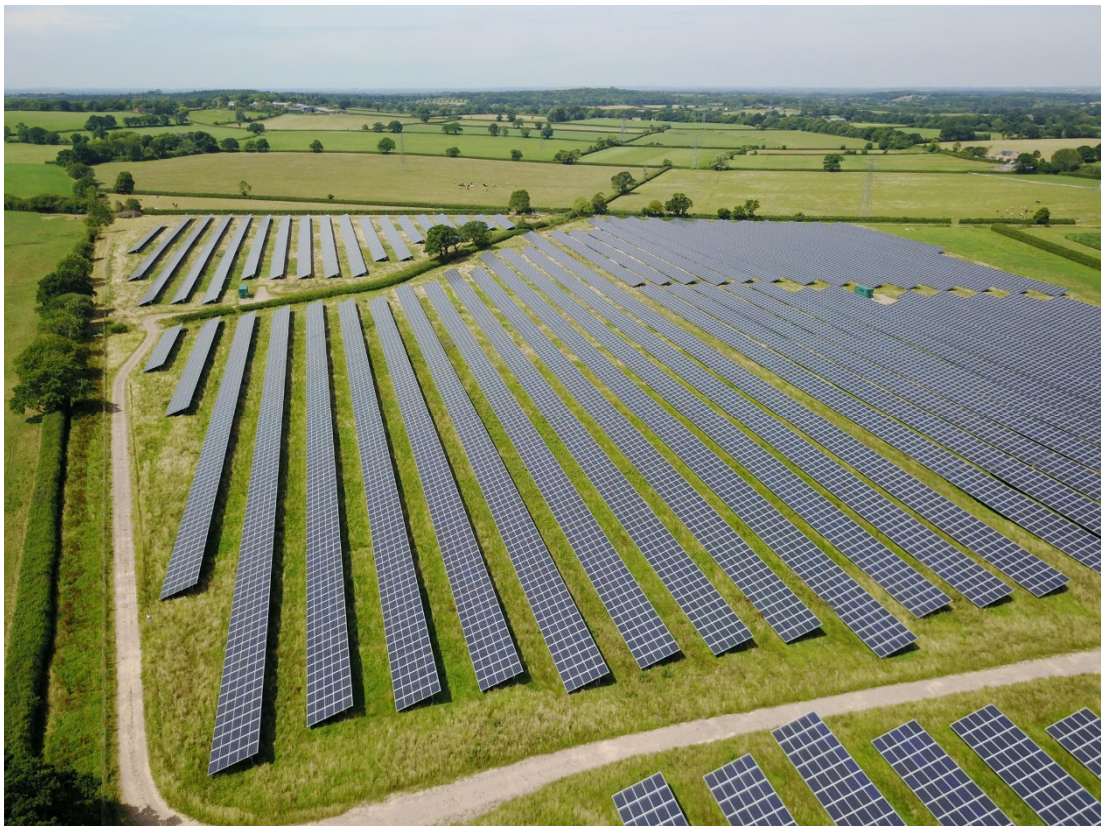
Fig. 1.11 - Aerial shooting of the "Braydon Manor" community-owned solar park [https://www.wwce.org/]
