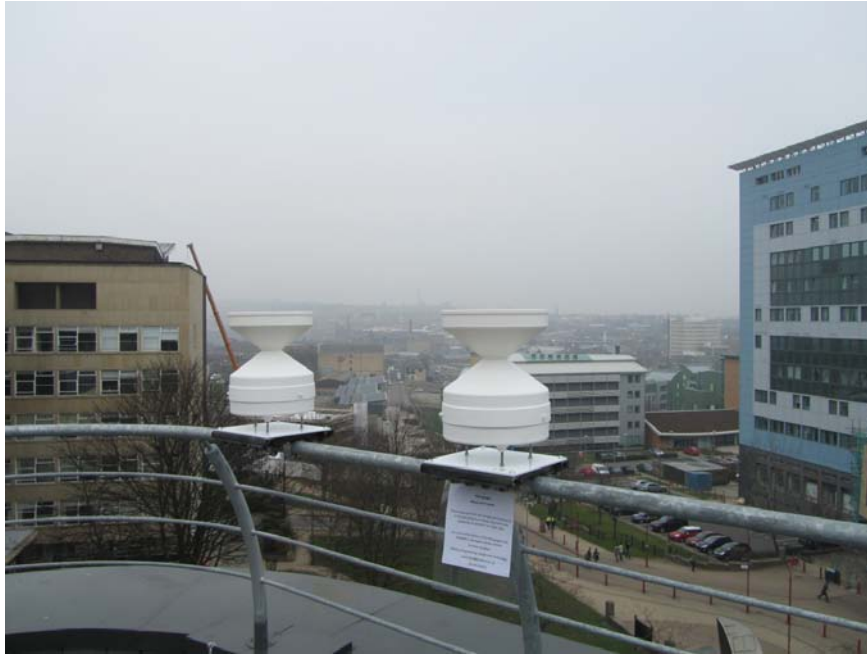
Figure 14: Rain gauges of point B, in School of Health.
