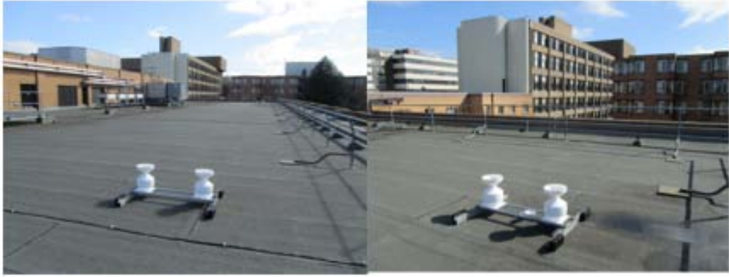
Figure 17: Rain gauges of point F and G, both in Library roof.
