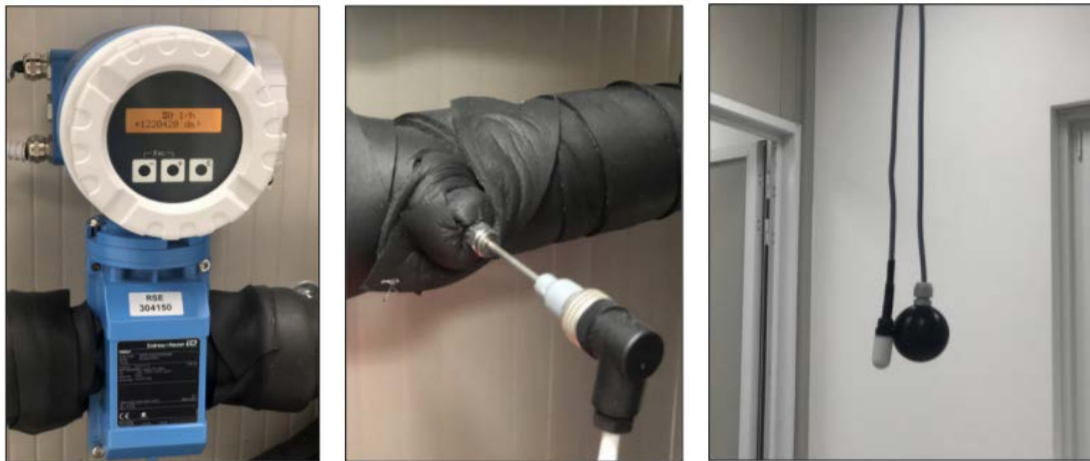
Figure 2.4: Water temperature probes (Pt100) of the fancoils system (left and center) and indoor temperature probe (right).
