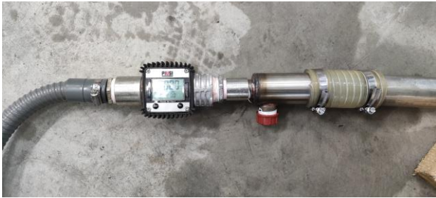
Flow meter installed on the draining pipe.
