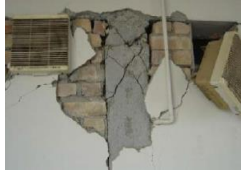
Short columns failure
