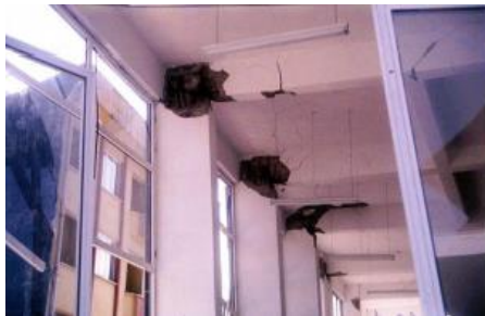
Joint shear failure
