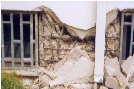
Short columns failure
