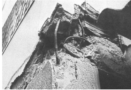
Figure 2.14: Exterior joint exhibiting Damage State 12
