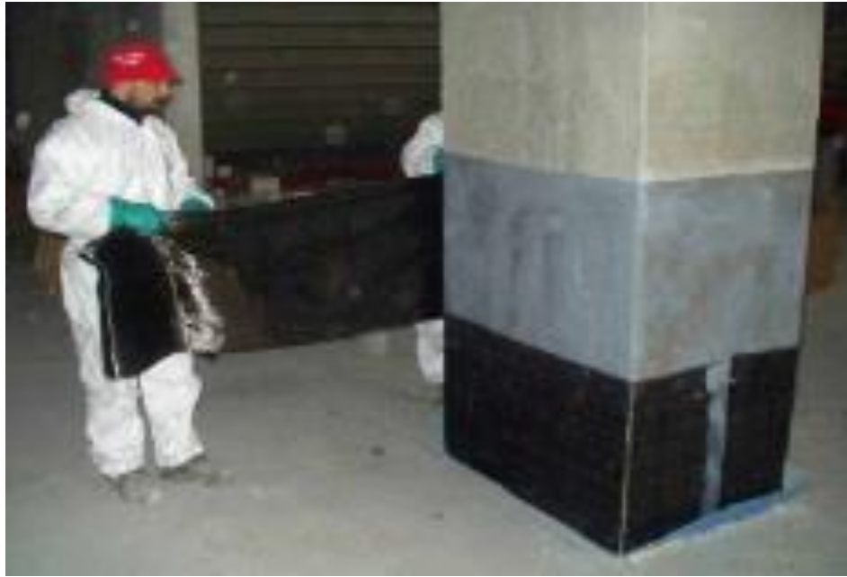
Figure 2.24: Application of CFRP fabrics to concrete columns for confinement of Reggio Emilia football stadium, Italy. (Book Composite for Construction, L.C. Bank)
