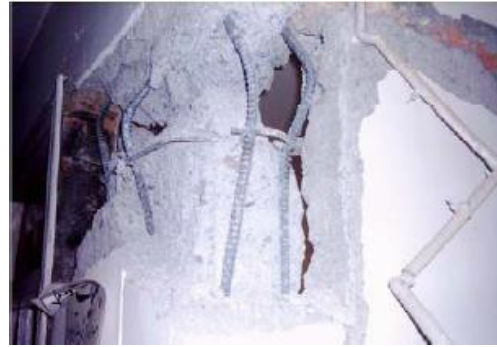
Local buckling in column
