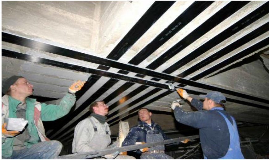
Figure 2.22: Flexural strengthening using CFRP strips of concrete girders in a Cement manufacturing building in Poland. (Book Composite for Construction, L.C. Bank)
