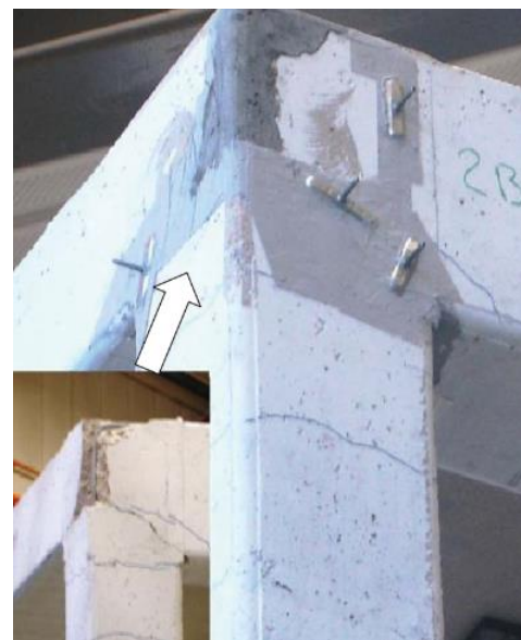
Figure 4.2: Mortar repair at second floor joint and injection ports for crack injection (Garcia et al. 2012)
