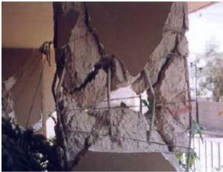
Shear failure in column
