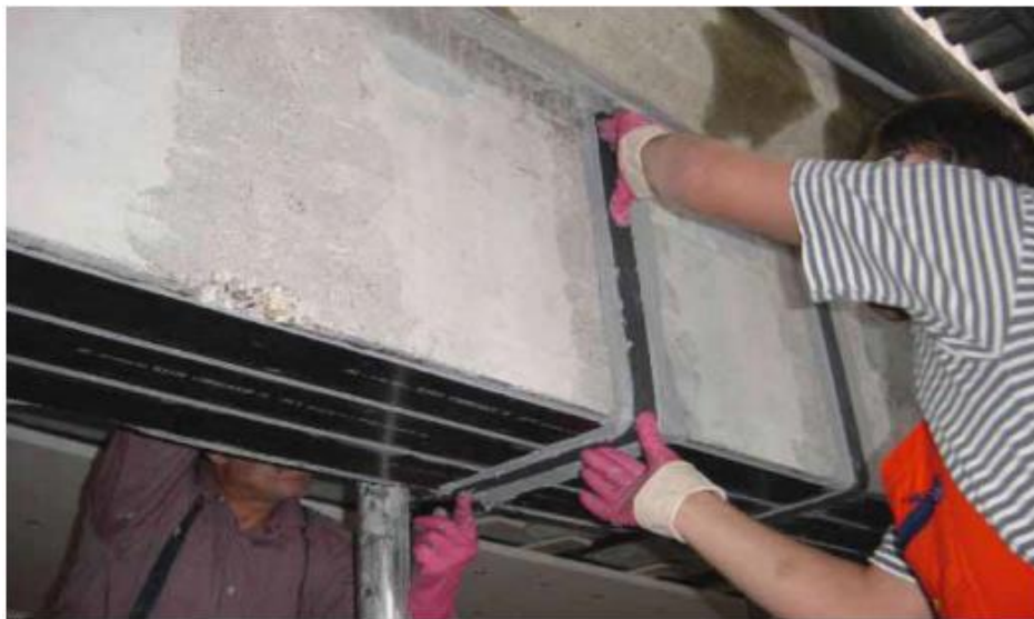
Figure 2.23: Installation of prefabricated CFRP L-shaped plates (shear strengthening) over existing CFRP strips (flexural strengthening). (Book Composite for Construction, L.C. Bank)
