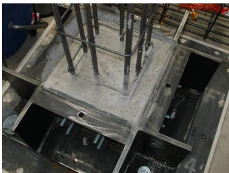
Figure 3.16: Specimen foot filled with concrete and ready for the formwork to be bolted (Garcia et al. 2012)
