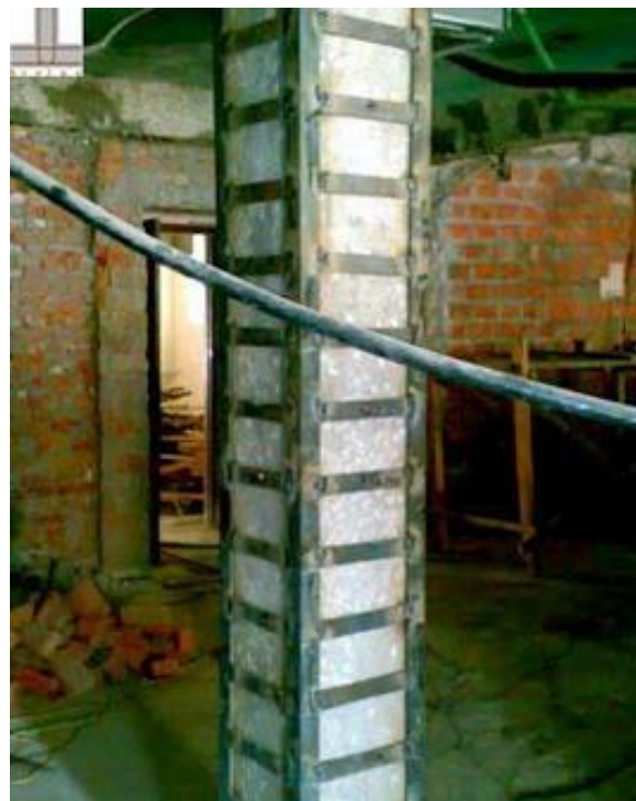
Figure 2.20: Retrofitting of the weak column using steel angles and bands (steel jacketing). Designed and applied by BREIN S Structural Care. Building Research Institute, Nepal.
