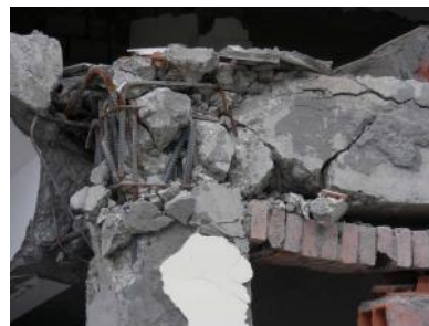
Inadequate joint confinement
