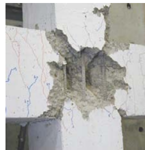
Figure 2.13: Joint specimen exhibits Damage State 11
