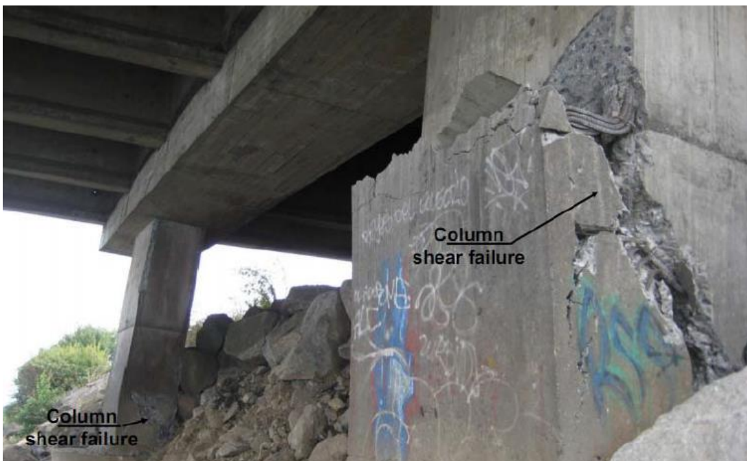
Figure 2.11: Juan Pablo II Bridge, shear failure of the columns [2].
