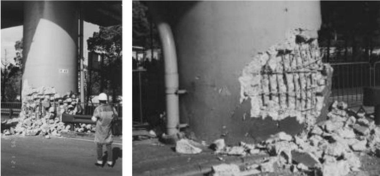
Figure 2.8: Flexural failure due to lack of confinement at the bottom of RC piers in Kobe earthquake, 1995 [3].
