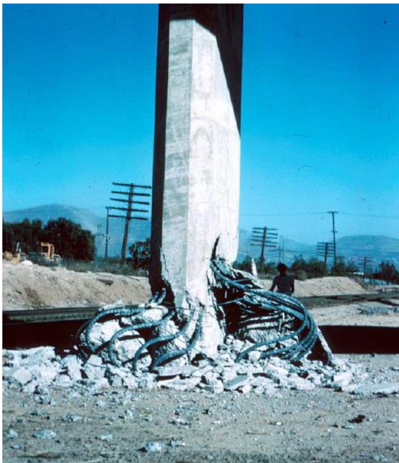
Figure 2.1: Damaged reinforced concrete column during San Fernando earthquake in 1971 [2].
