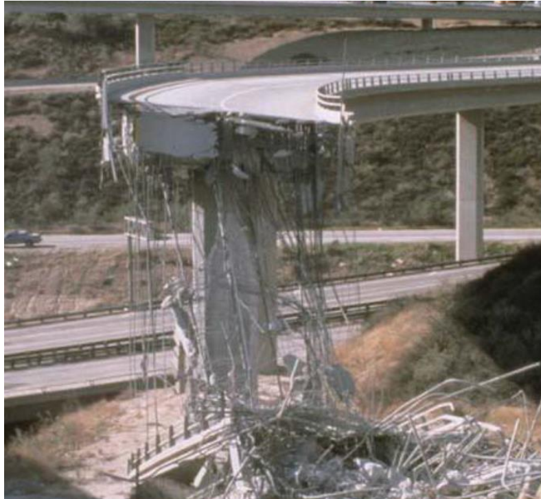
Figure 2.6: Span collapsed at the Golden State- Antelope Valley interchange collectors, due to the collapse of a column [3, 4].
