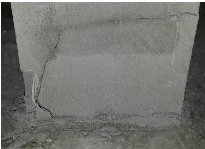
Figure 6.31: Cracking pattern obtained near the base of R/C column.
