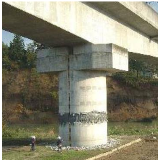
Figure 2.9: Damaged RC column of Unogawa Bullet Train Bridge [2].
