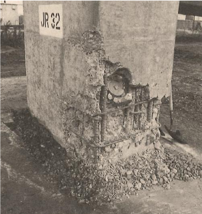
Figure 2.3: Failure at the bottom of a RC column after Loma Prieta earthquake, 1989[3].
