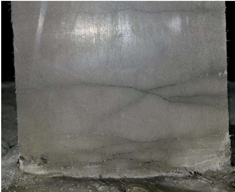
Figure 6.30: Formation of several cracks near the base of the Nitinol R/ECC column.
