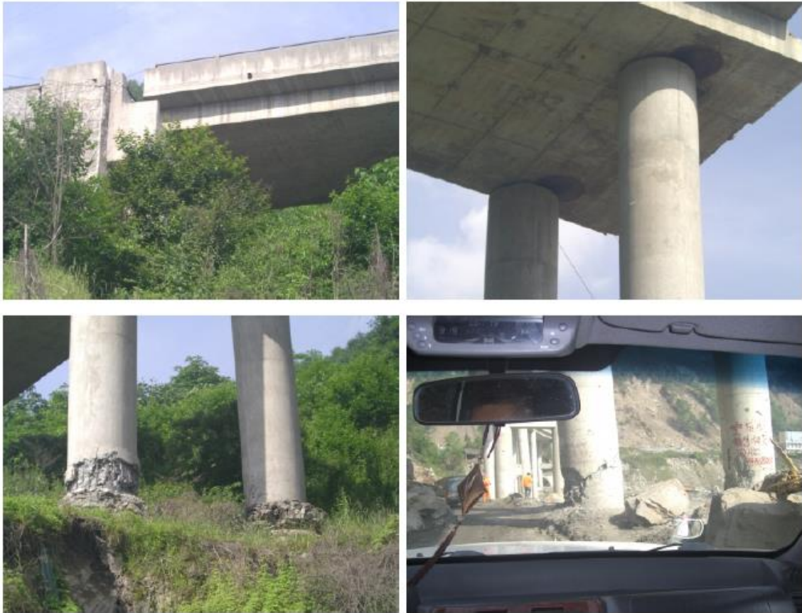
Figure 2.10: Damaged columns and relative displacements of joints on a bridge during Wenchuan earthquake [4].
