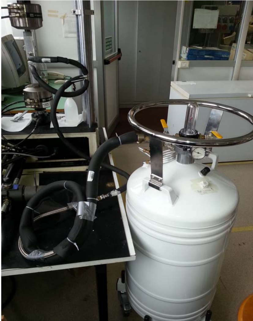
Figure 3.10: Refrigeration plant. The white cylinder on the right is the nitrogen Dewar; on the bottom left there are the ducts; on the left upper corner the clamp system is connected to the Teflon insulated pipes.
