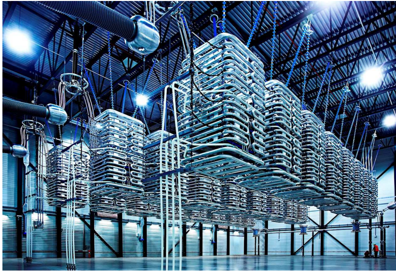
Figure 2.7: Example of HVDC (high voltage direct current) conversion station, build by ABB for a 400 MW DC Denmark-Germany interconnection [1]
