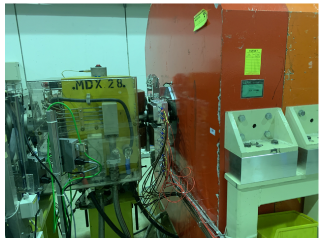
Figure 7.7: Picture of Veto Counter station 3 installed in the designed location.
