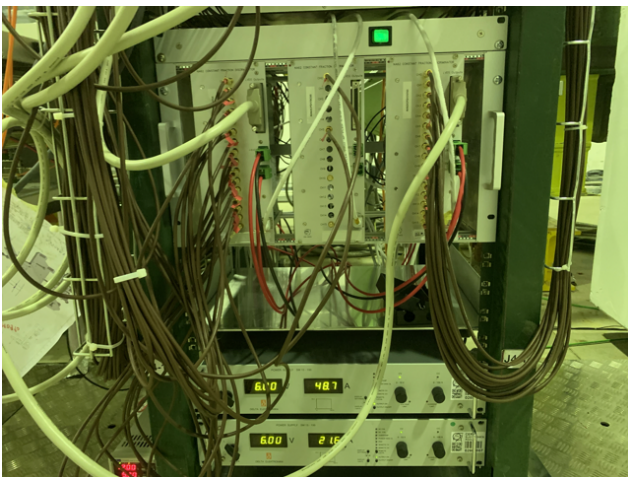
Figure 7.14: The CFD motherboards installed in the rack /2
